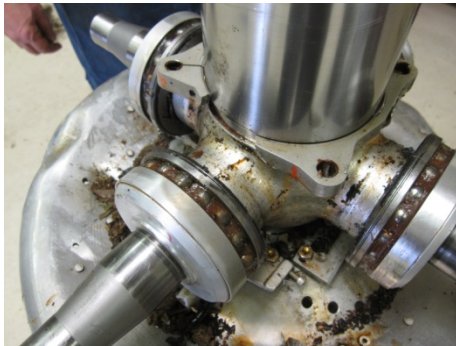
PHOTO 37: FRACTURED GUIDE COLLAR
