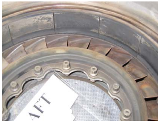
PHOTO 19: LIGHT CONTACT SCORING ON THE 1 ST -STAGE TURBINE BLADE TIP SHROUDS
