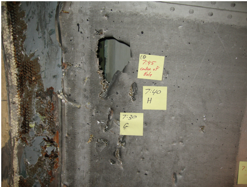
PHOTO 8: INLET COWL INNER BARREL DAMAGE - LOCATIONS 3 AND 4
