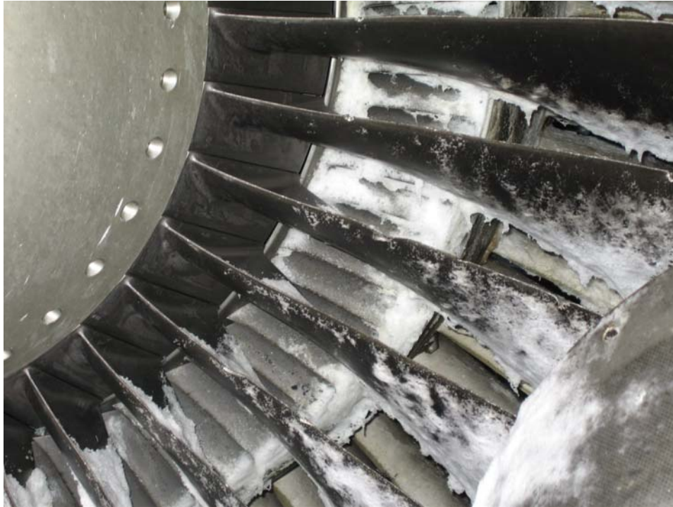
PHOTO 20: NO DIRT OR EARTH DEBRIS INGESTED
