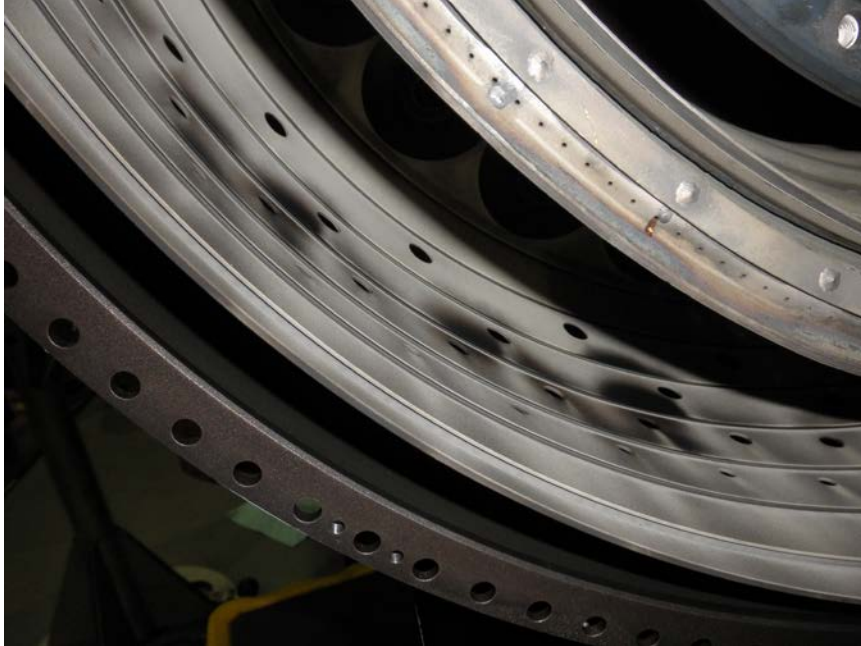
Photo No. 14: View of the combustor outer liner showing random sooting.
