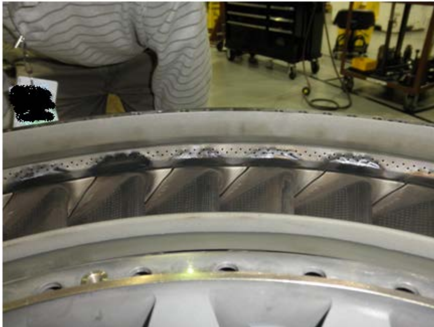
Photo No. 17: Close up view of the 1st stage turbine vanes showing dark discoloration on airfoils and light-colored areas on outer platforms.
