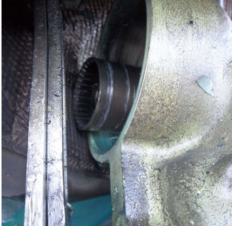
Figure 16. Muff coupling exposed
