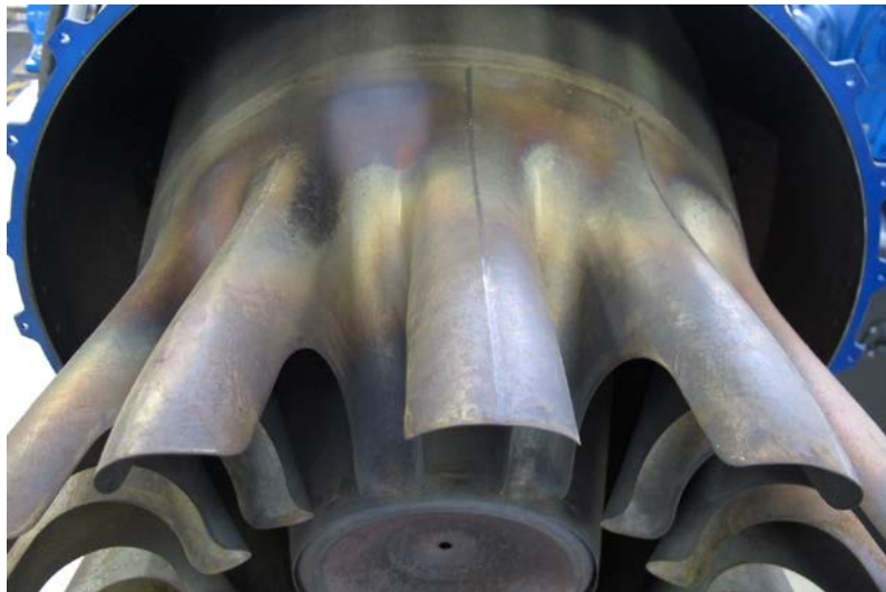
Photo 7- Exhaust Mixer Lobes, Mild Discoloration and Sooting
