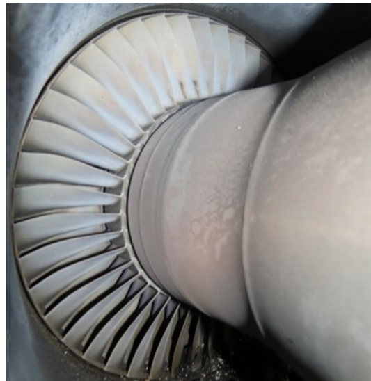
Figure 50. PT rotor viewed through the exhaust
