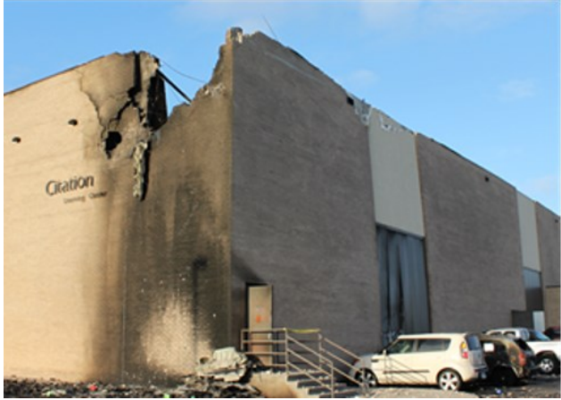
Figure 1. Initial point of impact
