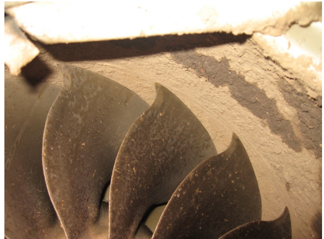
PHOTO 12: FAN CASE FLOW PATH WITH THIN LAYER OF DIRT
