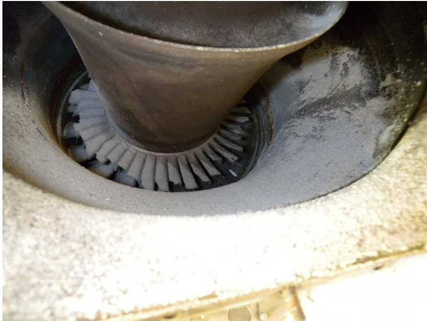
Figure 5 – Power Turbine Wheel – All Blades Fractured
