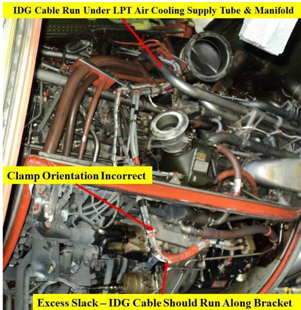
PHOTO 39: MISROUTED IDG POWER FEEDER CABLE ON EVENT ENGINE
