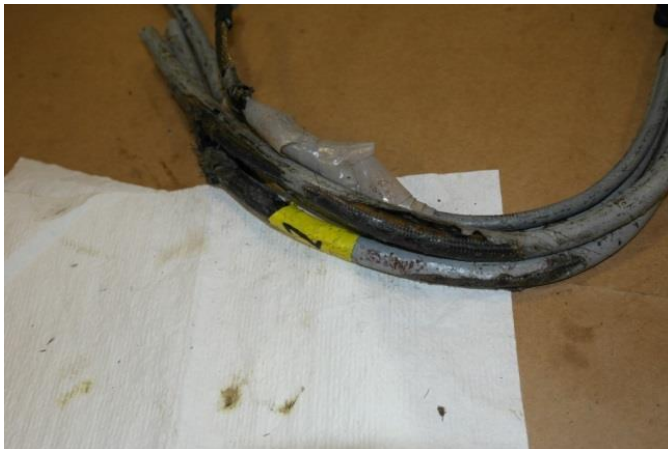
PHOTO 24: THERMAL DISTRESS TO IDG POWER FEEDER CABLES
