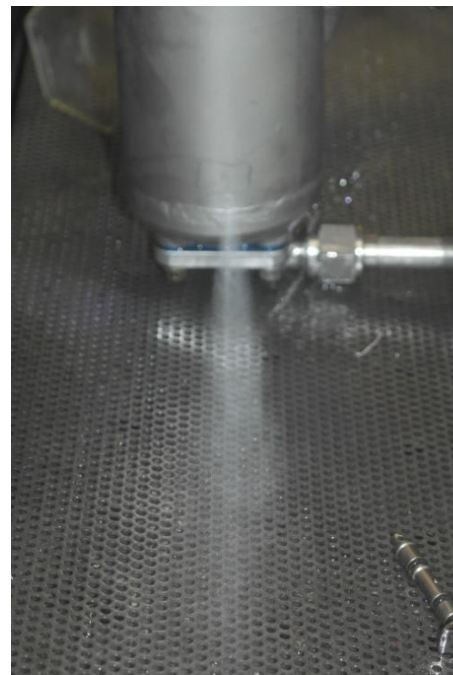
PHOTO 22: LEAK AT 400 PSI FLUID PRESSURE
