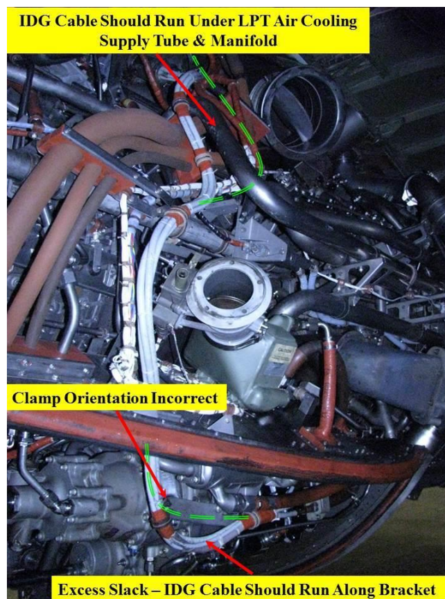
PHOTO 38: MISROUTED IDG POWER FEEDER CABLE FOUND DURING THE FLEET INSPECTION
