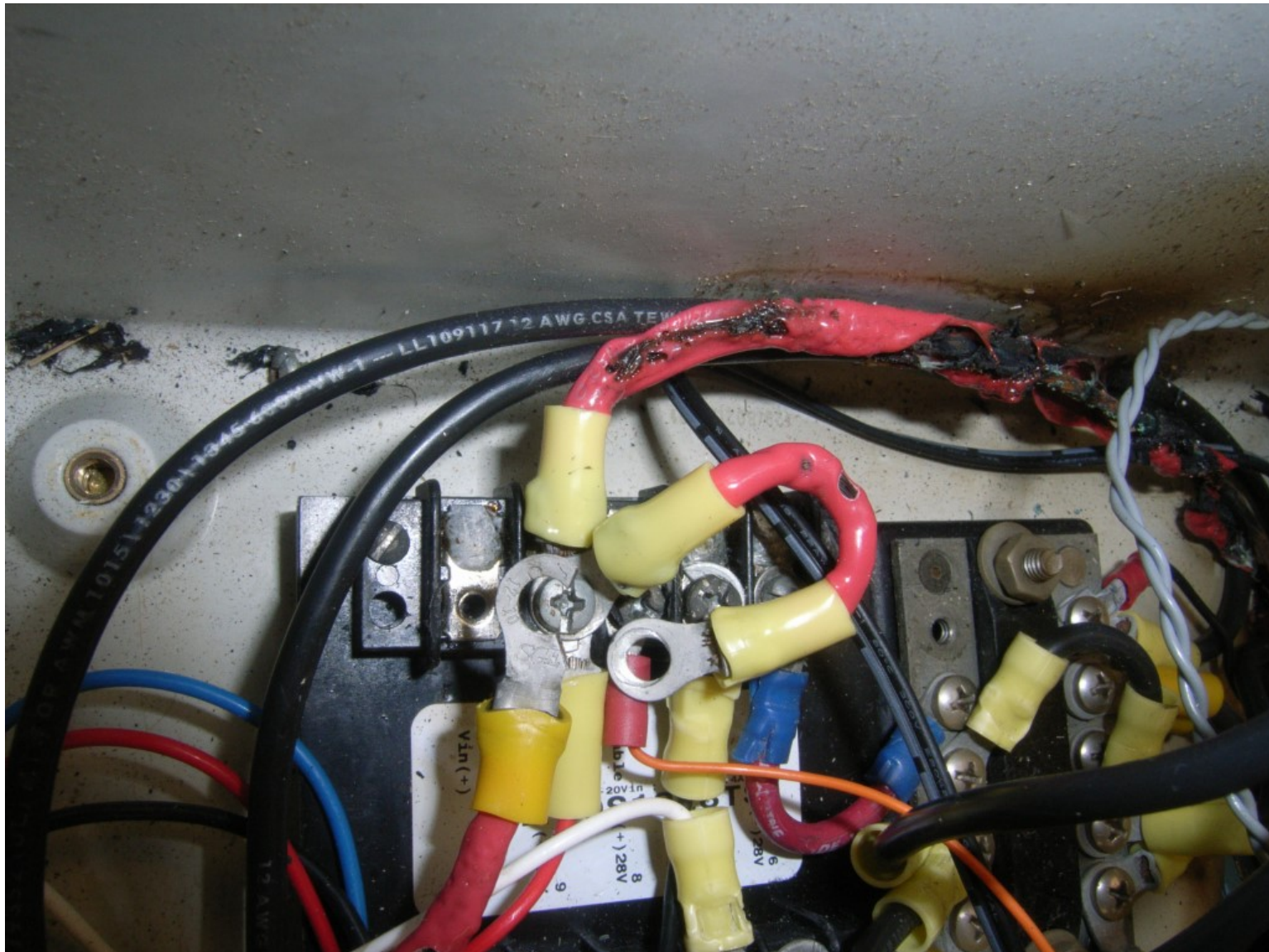
Figure 9 - Step Up Transformer and Bus Block
