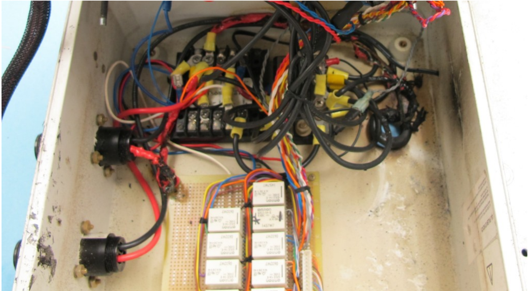
Figure 5 - Interior View of Power Distribution Box (Looking forward)
