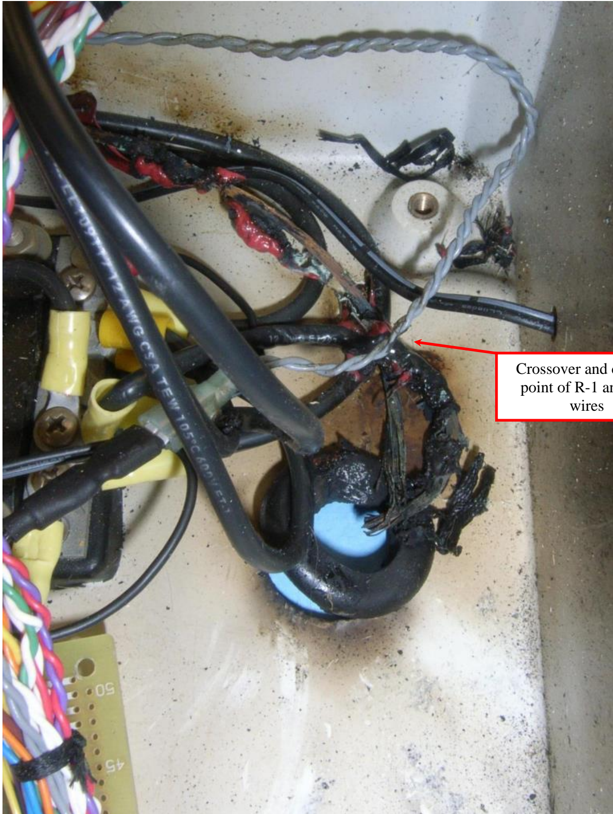
Figure 10 - Grommeted Hole and Damaged Wires
