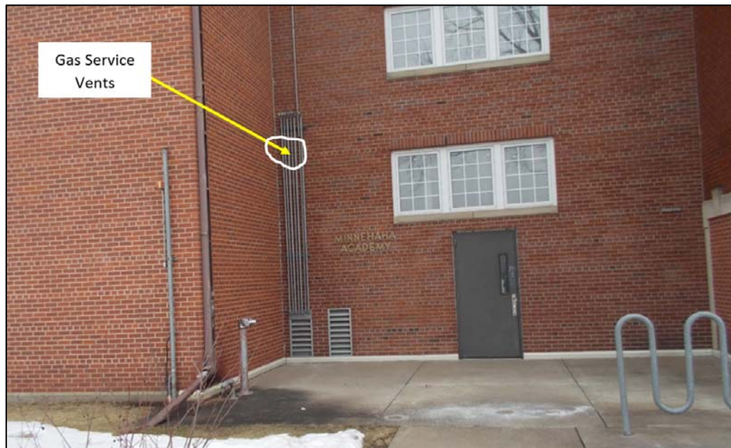
Figure 3 – Sidewalk over utility bunker (gas meter room) at the rear (west end) of the Minnehaha Academy building showing gas vent pipes. Source: CPEMG, taken: Feb2016
