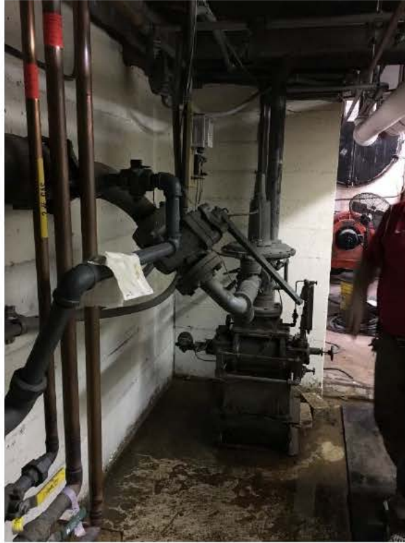
Figure 4 – View from utility bunker (gas meter room) into boiler room. Source: CPEMG, taken Feb 2017
