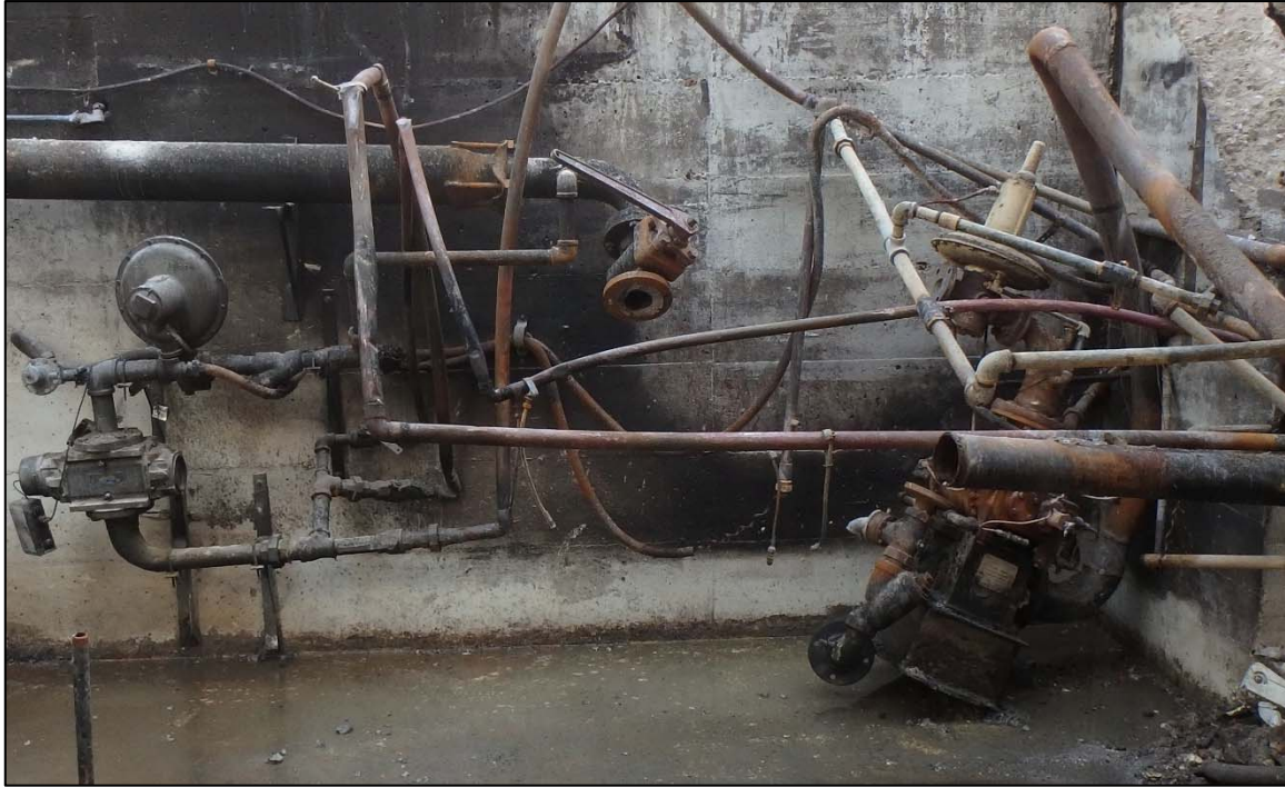
Figure 10 – Plug valve handle positioned perpendicular to the direction of gas flow. Source: NTSB, Taken: 6Aug2017
