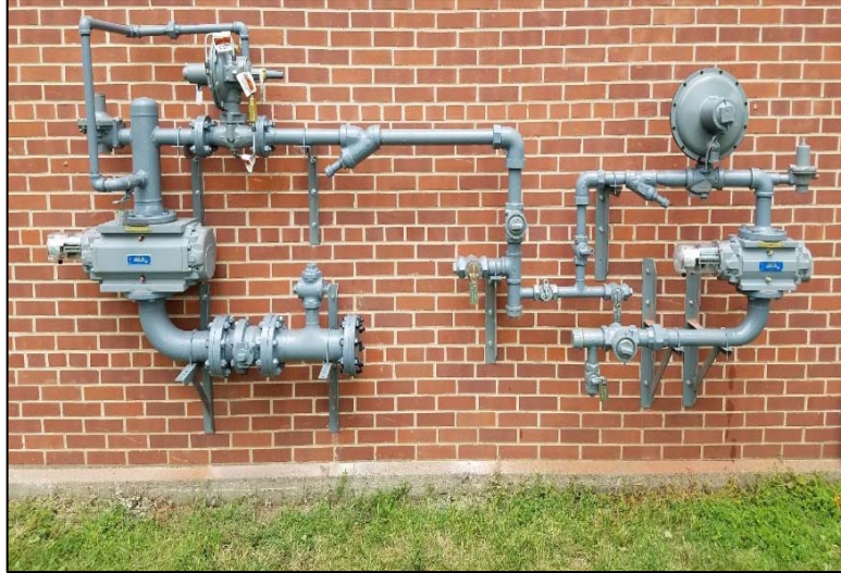
Figure 8 – Two new gas meters assemblies mounted on the west rear wall of the Minnehaha Academy building by CPEMG on June 29, 2017; the planned new location. Source: CPEMG.
