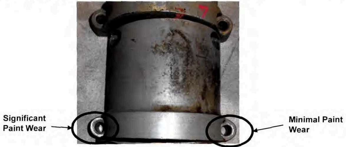
Clamp "A" wear at bolted joint interfaces.
