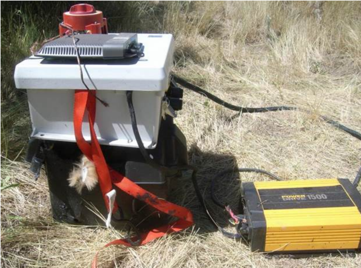
Stackup of Battery, Distribution Box, and Modem & Switch plus yellow inverter (view from airplane right)
