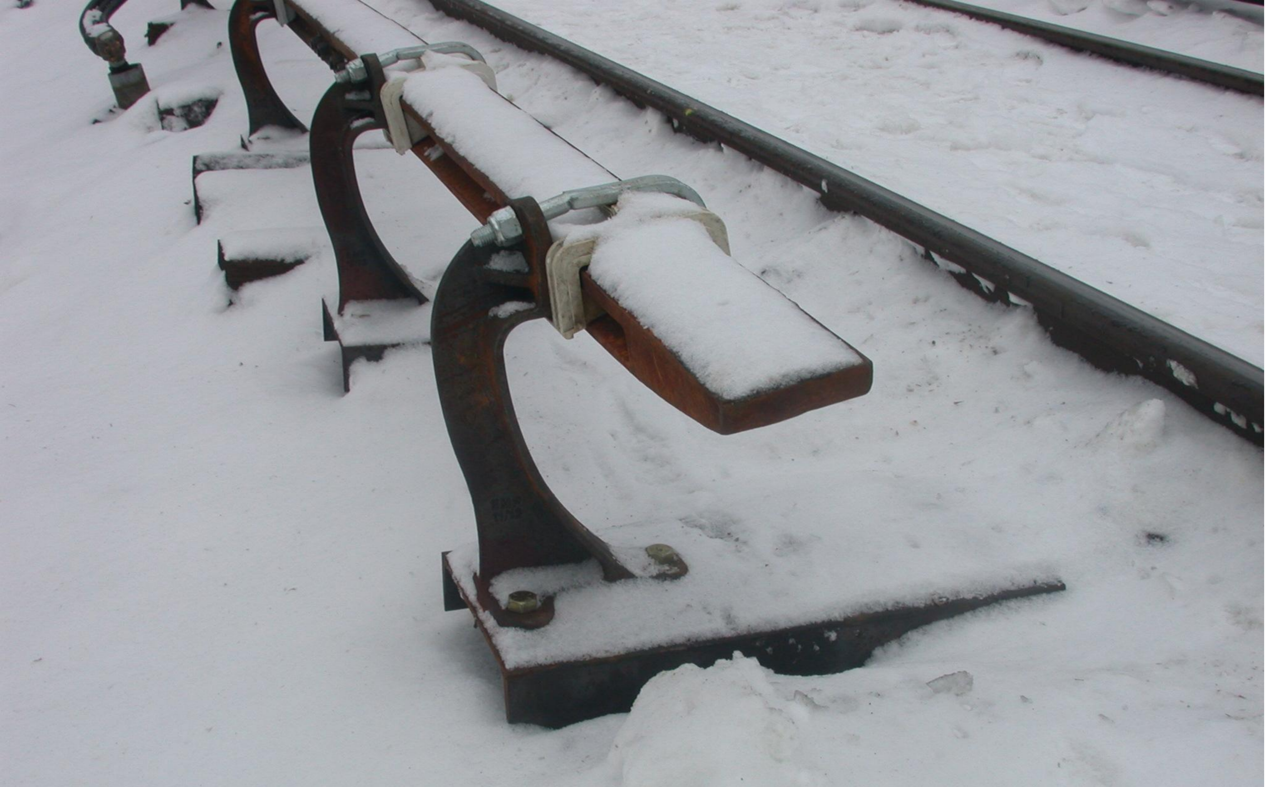
View of the 3rd rail nose piece installed on the west side of main track 2
