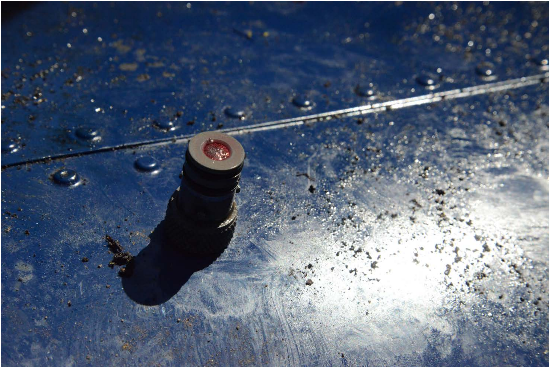
Photo 12 - View of the removed magnetic plug from the hydraulic system.
