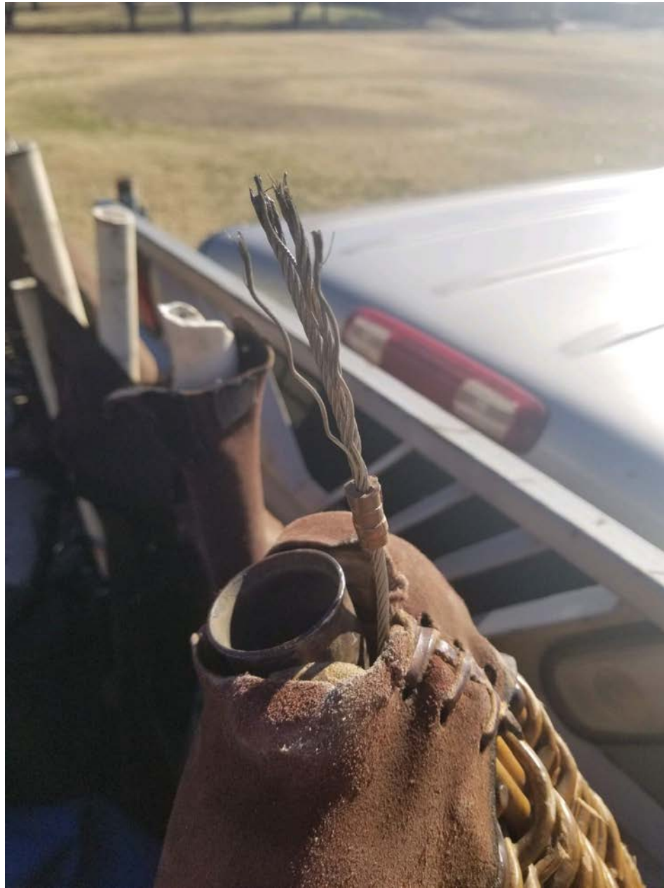
Photo 2 – View showing one Broken Suspension Cable
