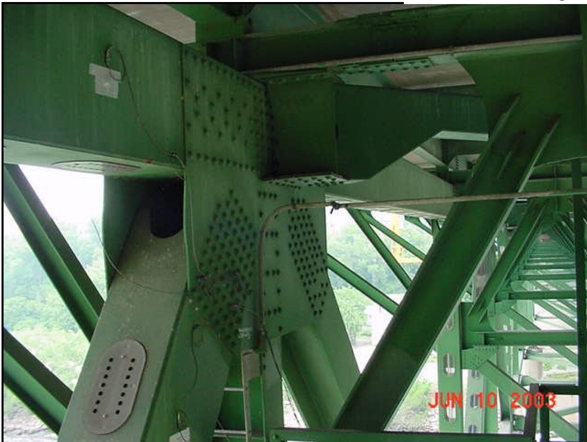
Node U10 West, viewed looking northwest from inside the structure.
