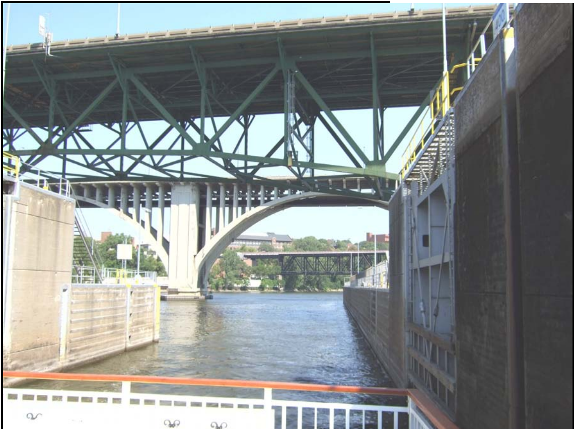
Looking east at the center span of the deck truss from a boat in the lock on July 31, 2007.
