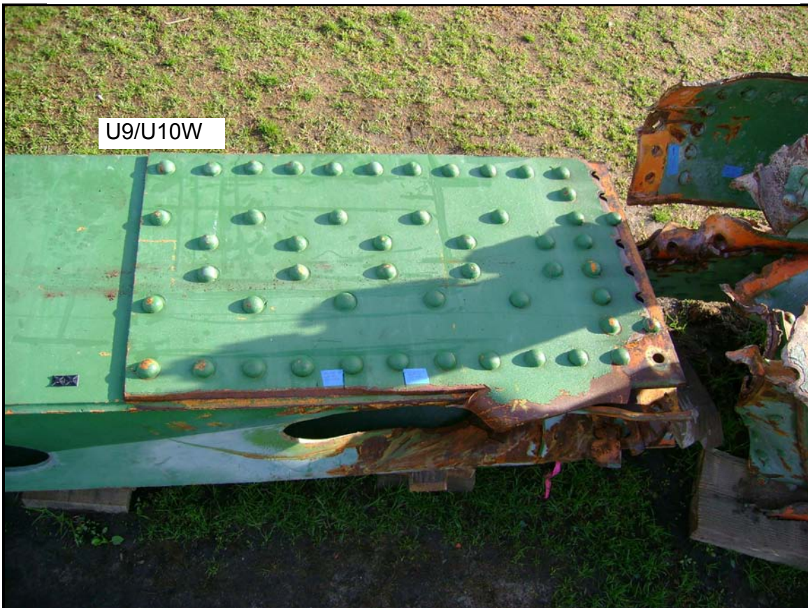
Node U10 West, showing the portion of the east gusset plate on U9/U10W.
