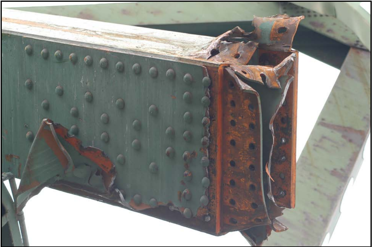
The end of U9/U10'W, showing the fractured west gusset plate.
