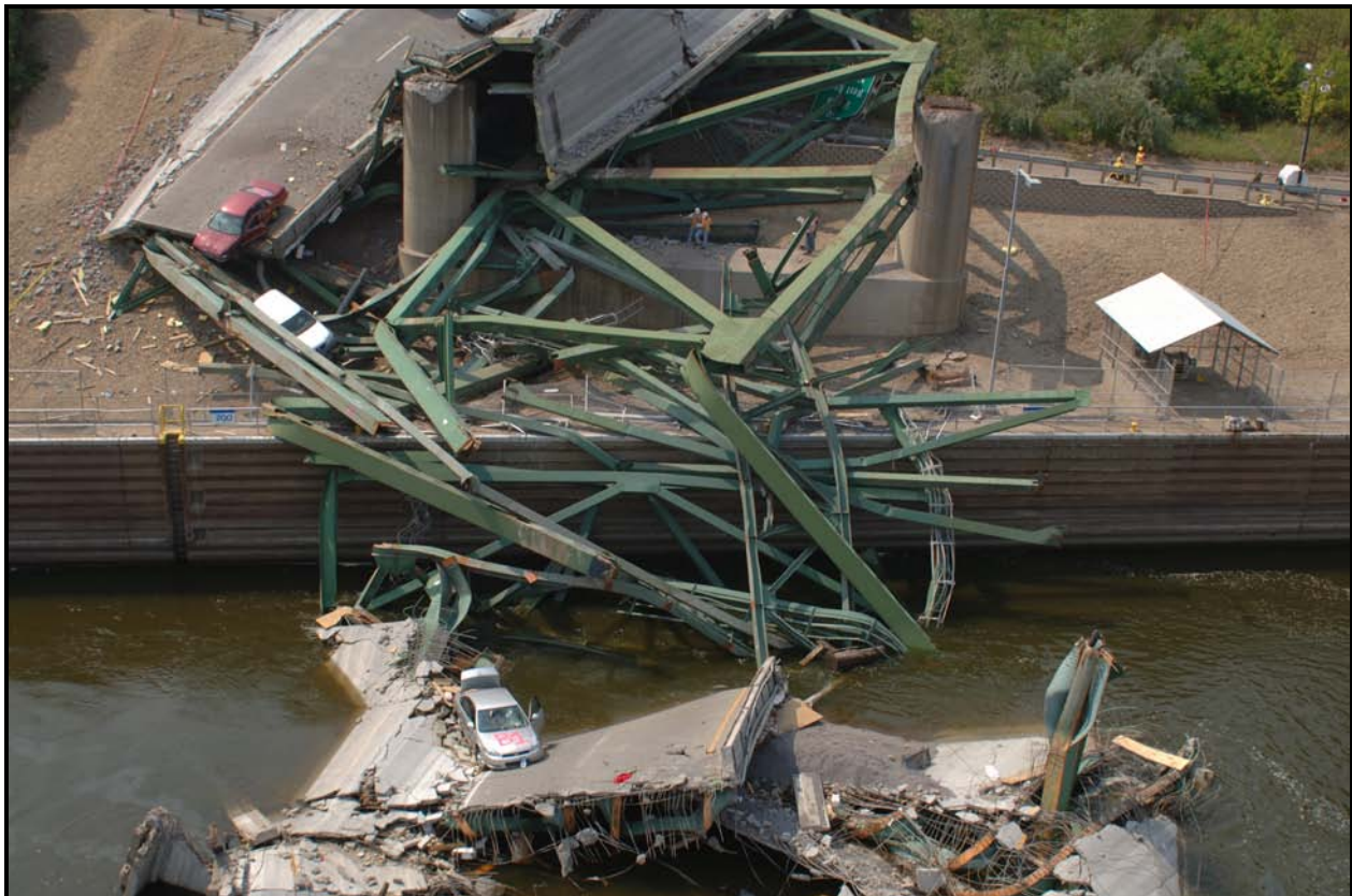
Deck truss structure on the south bank of the river, viewed looking south.
