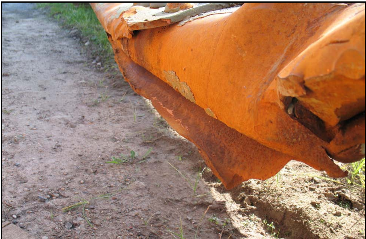
Node L11 West, showing corrosion adjacent to the fracture in the west gusset plate.
