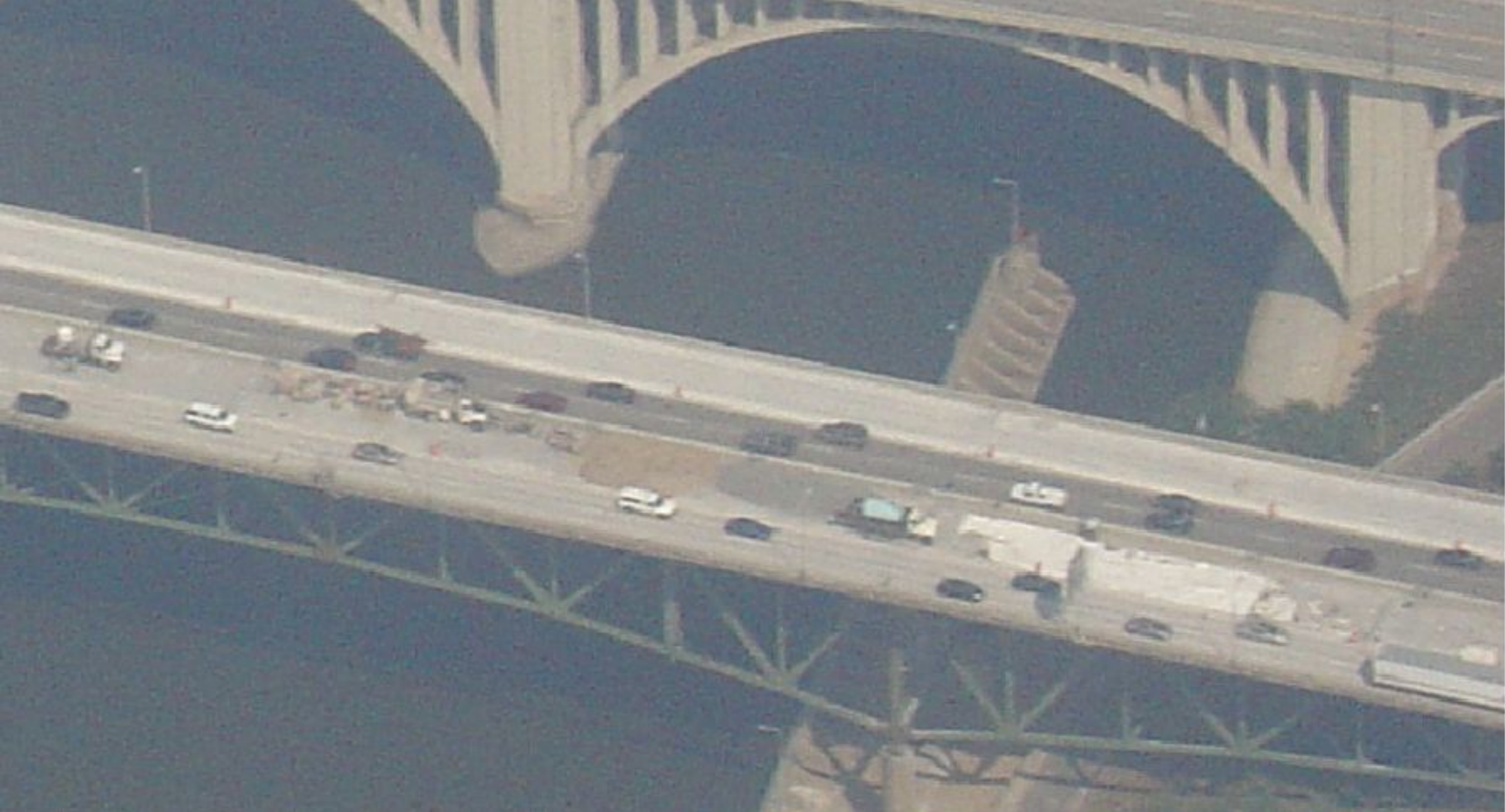
Photograph of Aggregates on Bridge Deck
