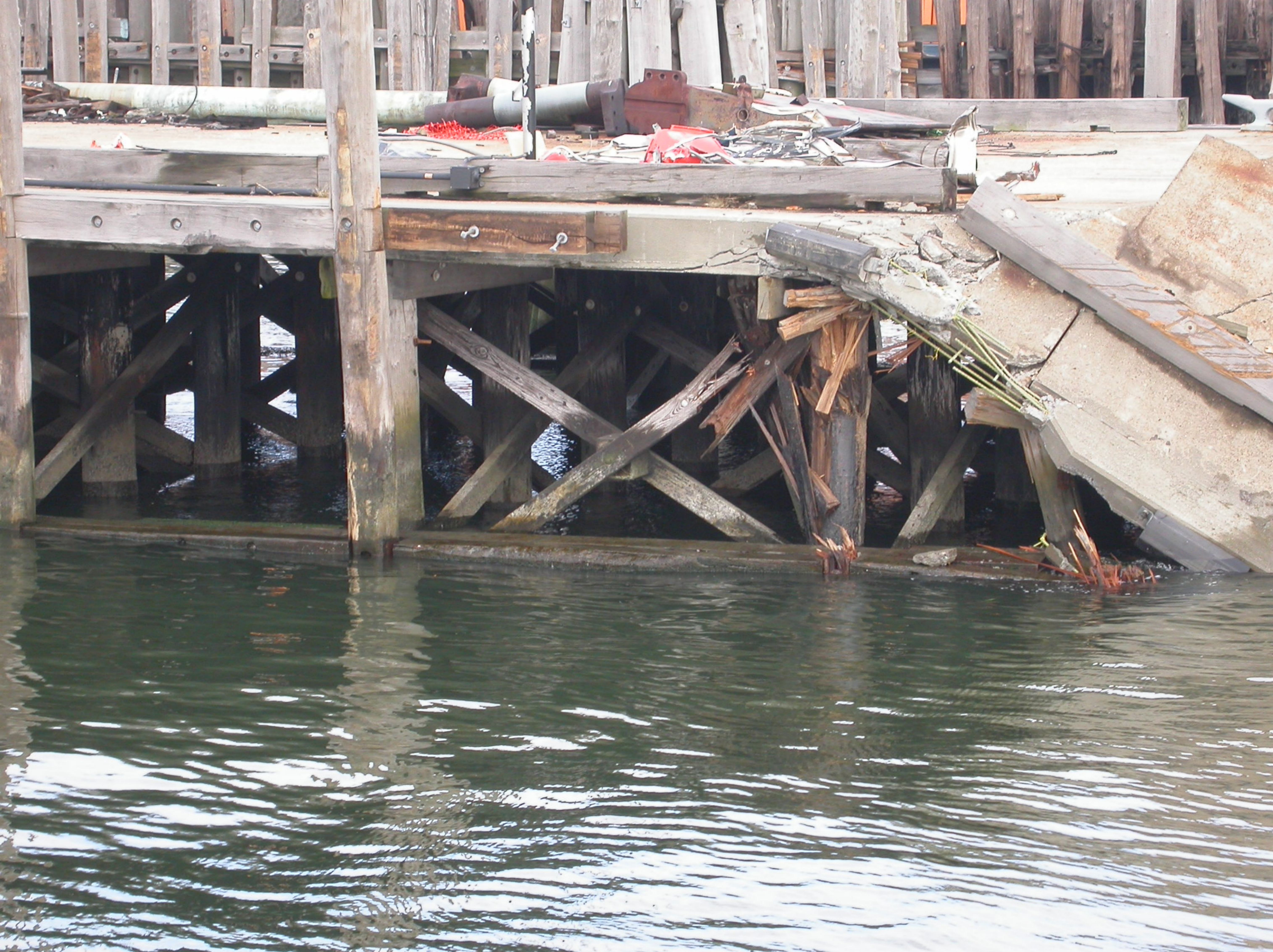
Photo of pier damage
