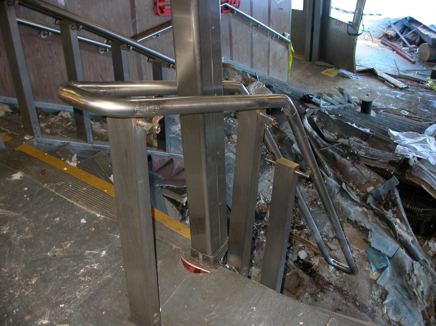
Photo of damaged stairwell, Staten Island end
