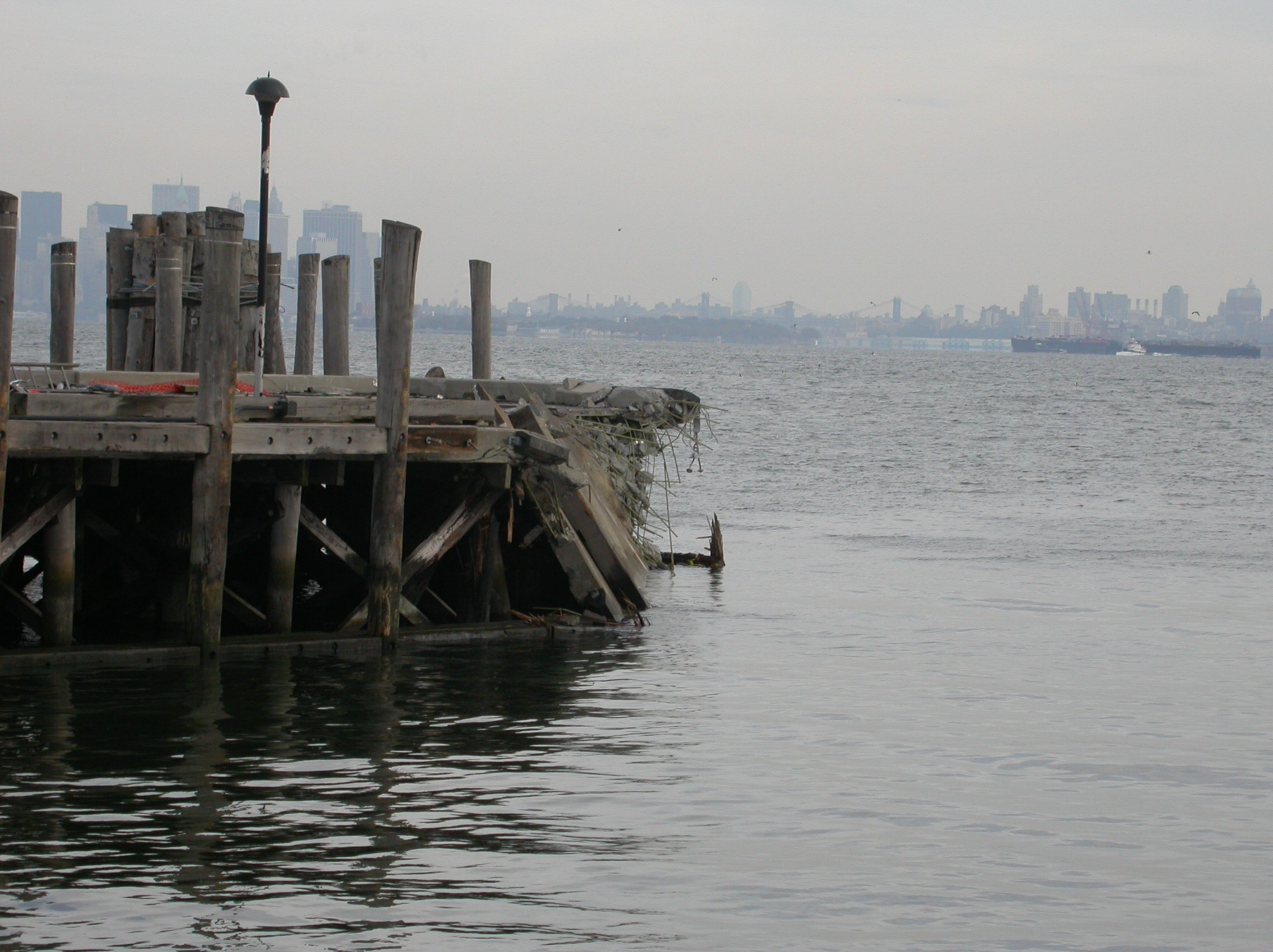
Photo of Pier damage
