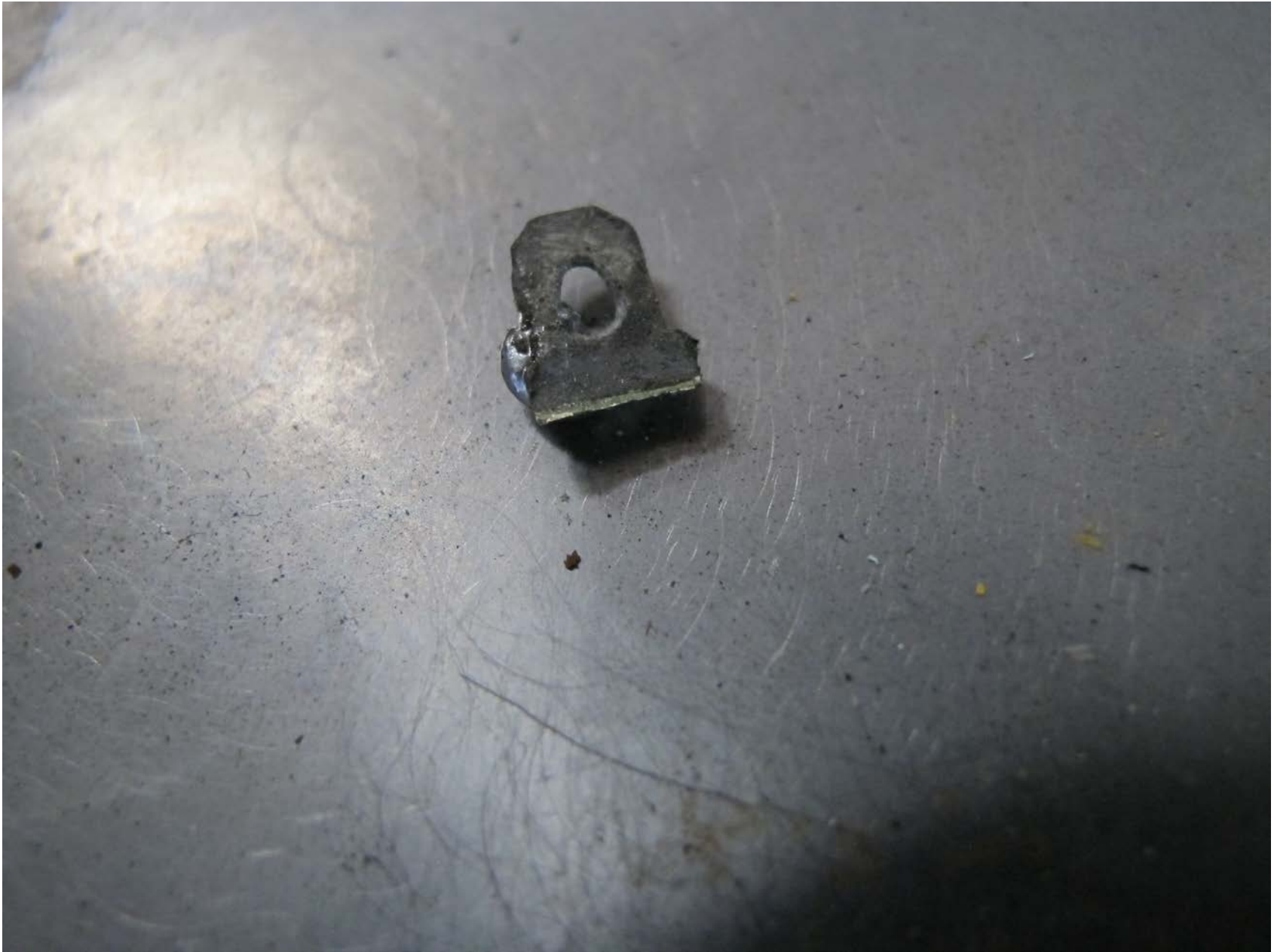
Photo 15 – Terminal of fuse holder (RH Photo)
