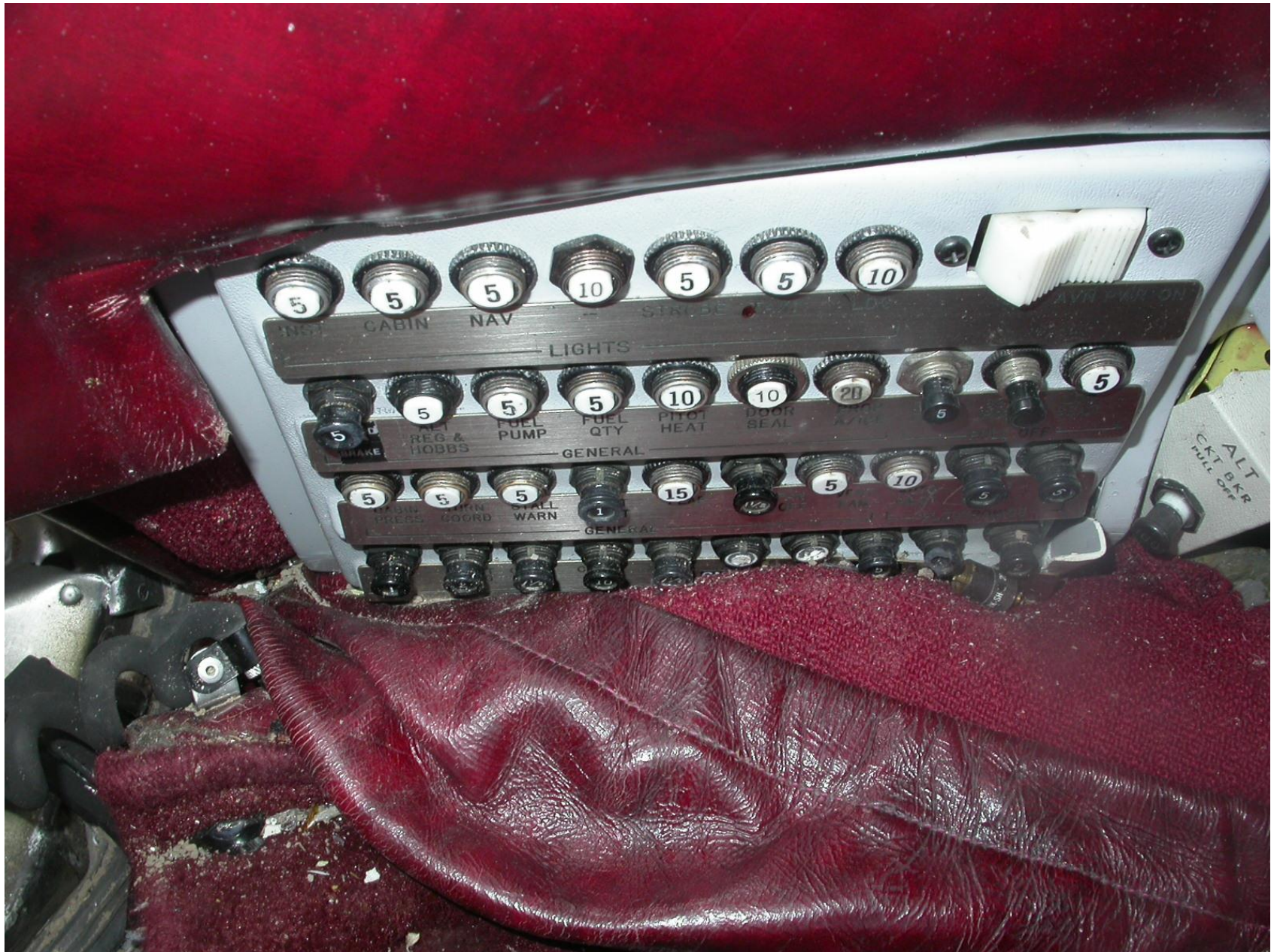
Photo 11 – View of circuit breaker panel
