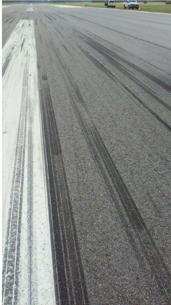
Photo 1 – Skid Marks Right of Centerline (Courtesy FAA)
