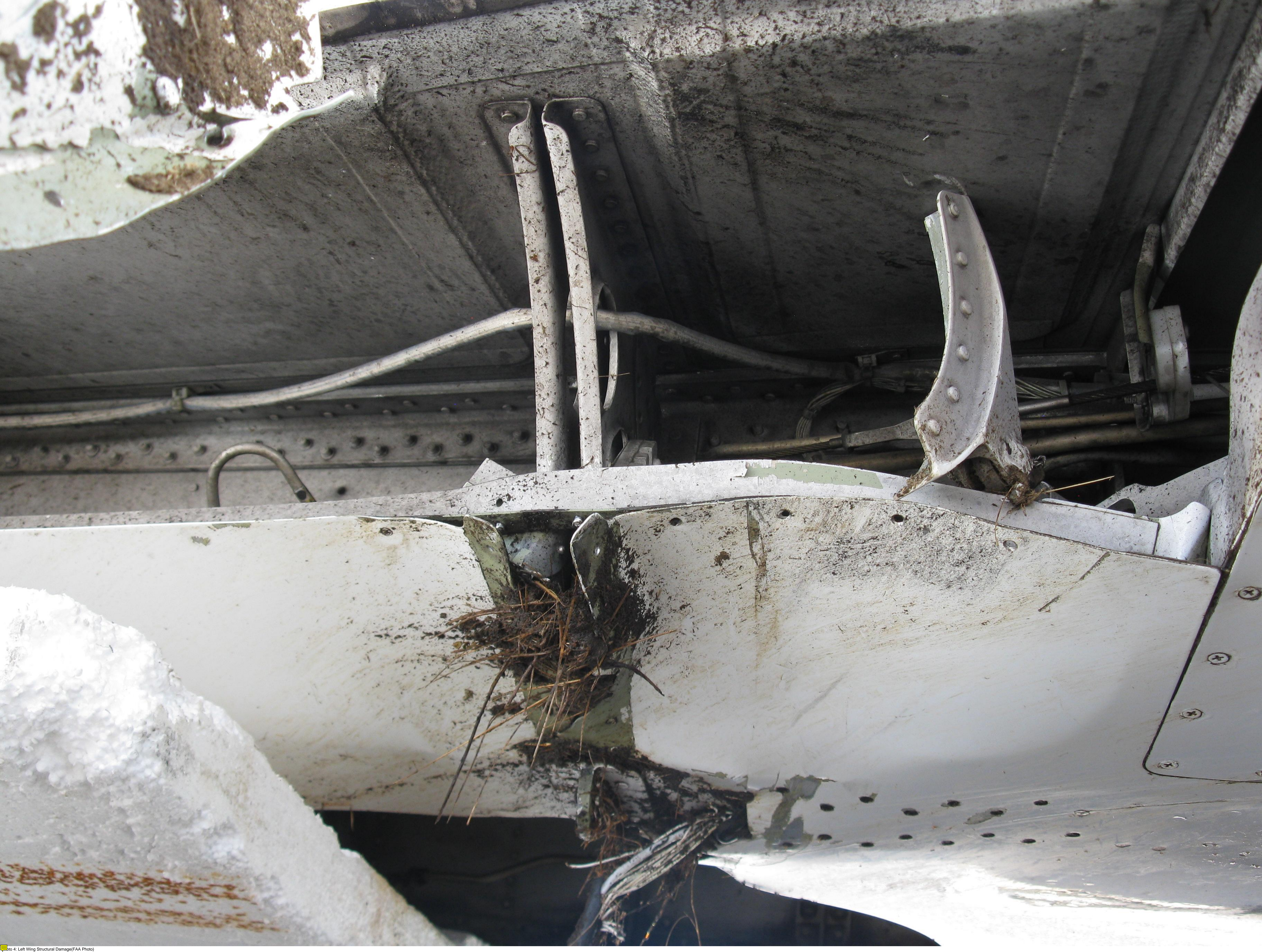
Photo 4: Left Wing Structural Damage (FAA Photo)
