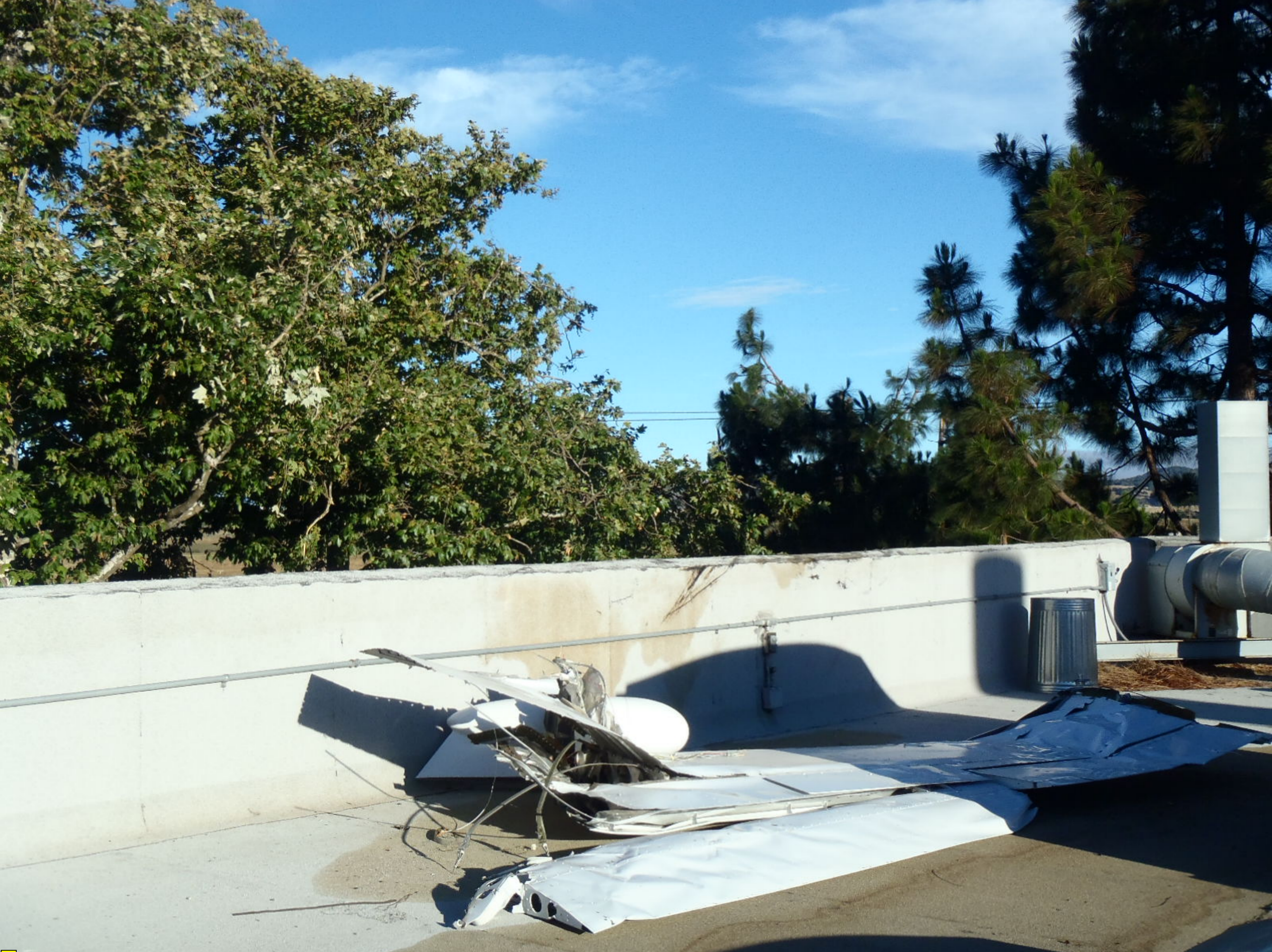
Photo 3 - Tree Damage at Accident Site
