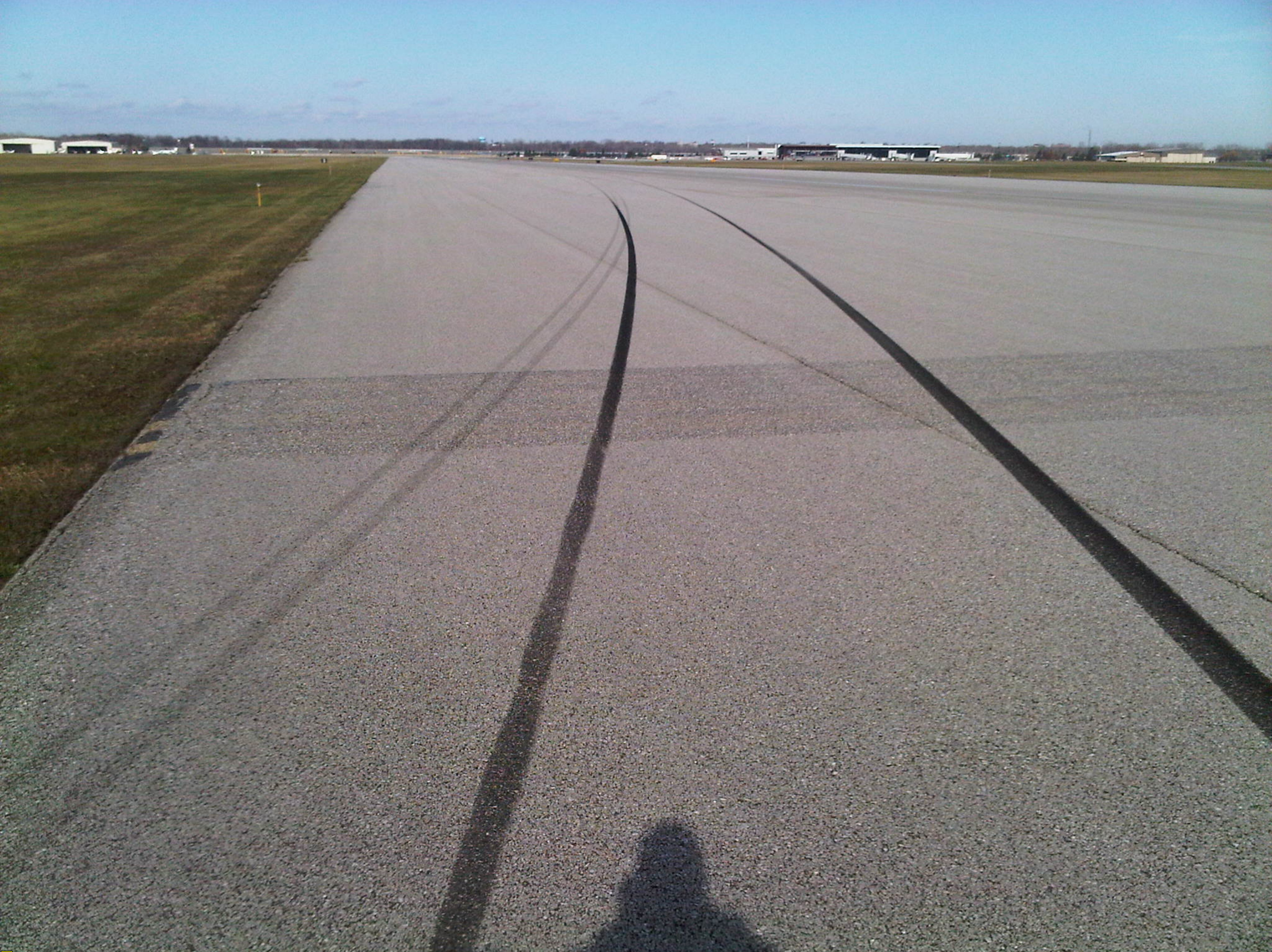
Photo 2 View of Runway Tire Skid Marks
