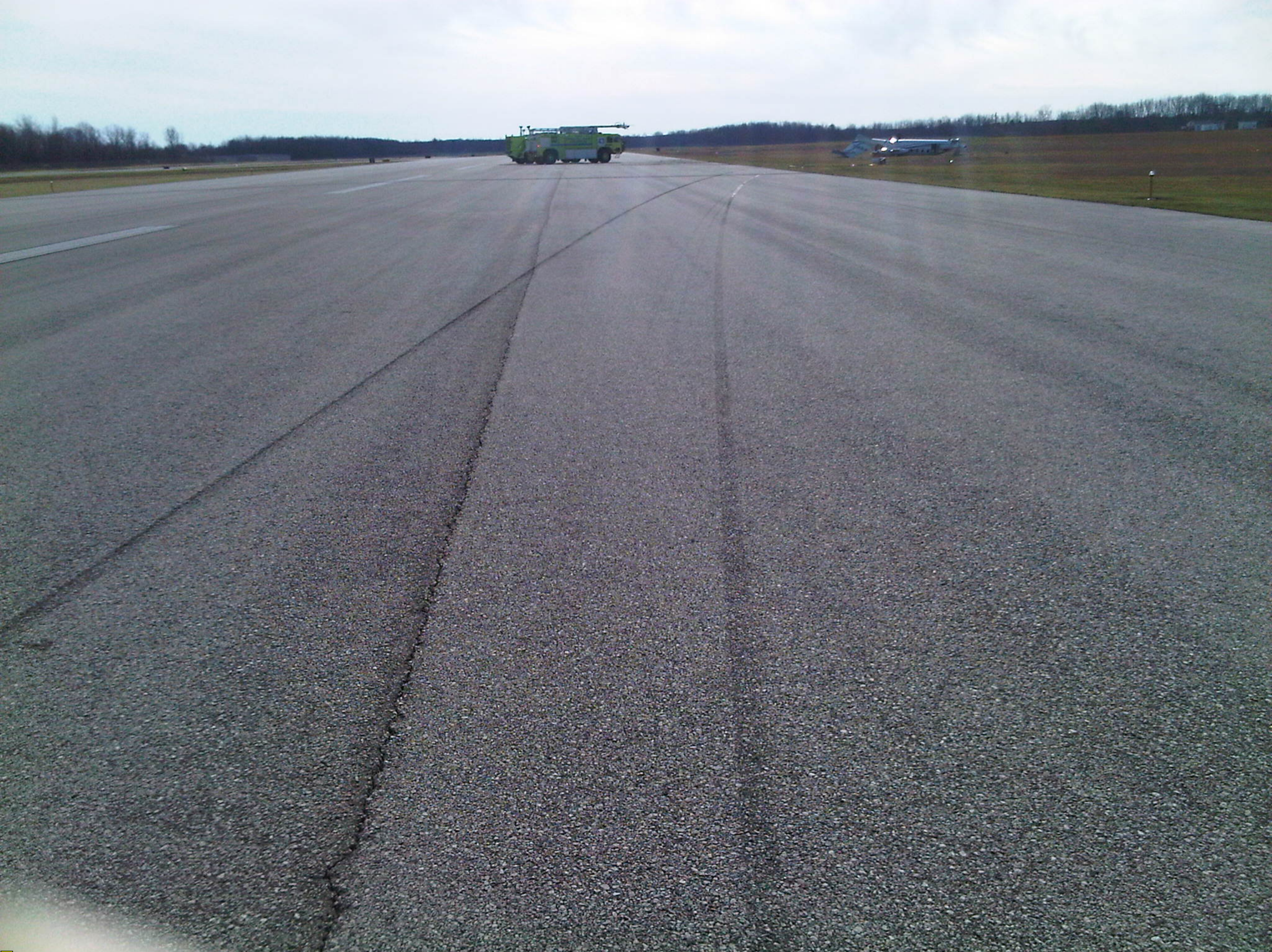
Photo 1 - View of Runway Tire Skid Marks
