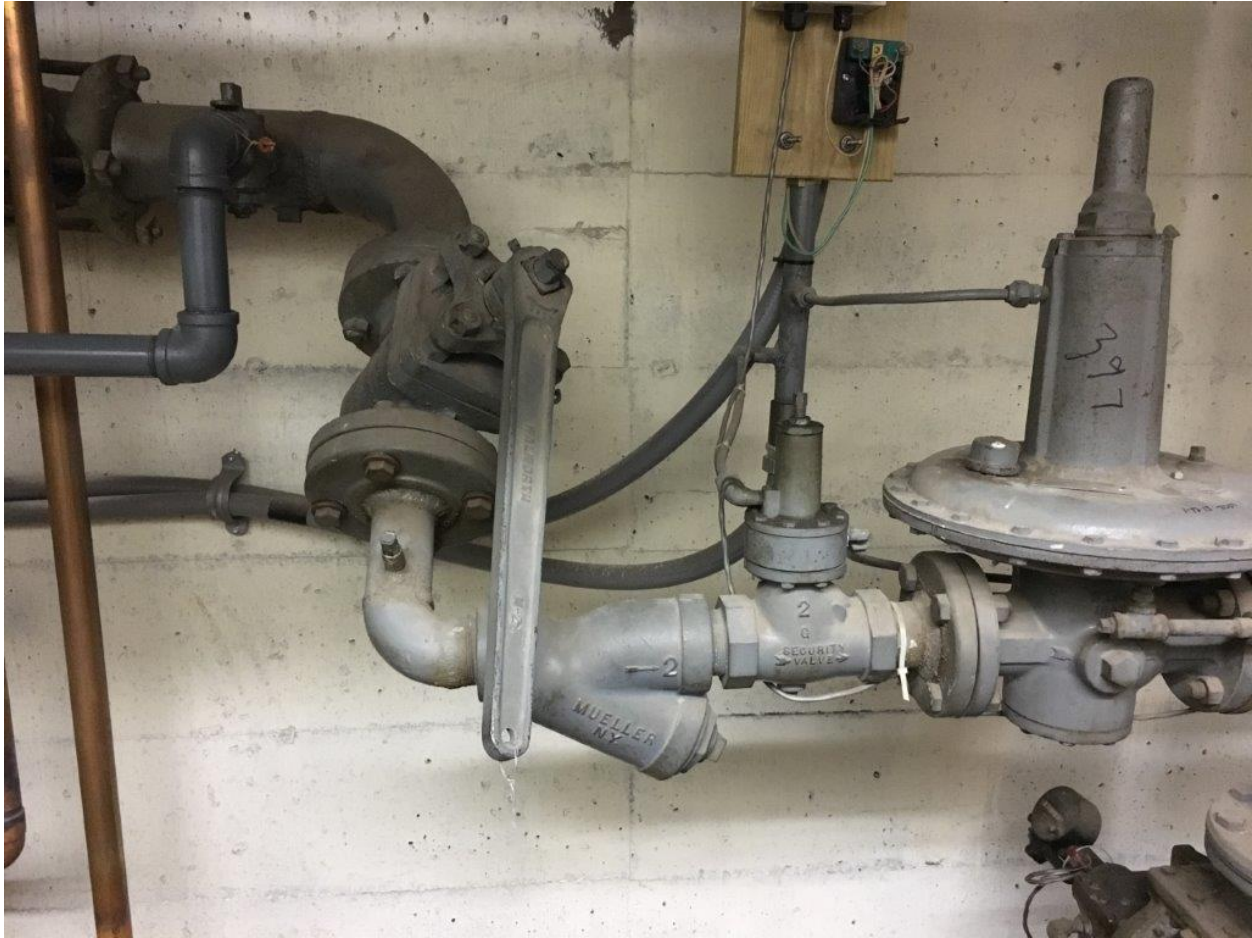
Figure 4: February 2017 photograph taken by CPEMG
