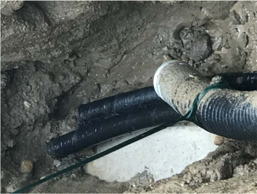
Figure 16: The exposed end of the three flow lines under the removed concrete slab. The 1” line is underneath the exposed two 2” line
