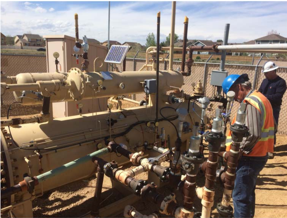
Figure 6: End of active 2" flowline at oil water separation unit.
