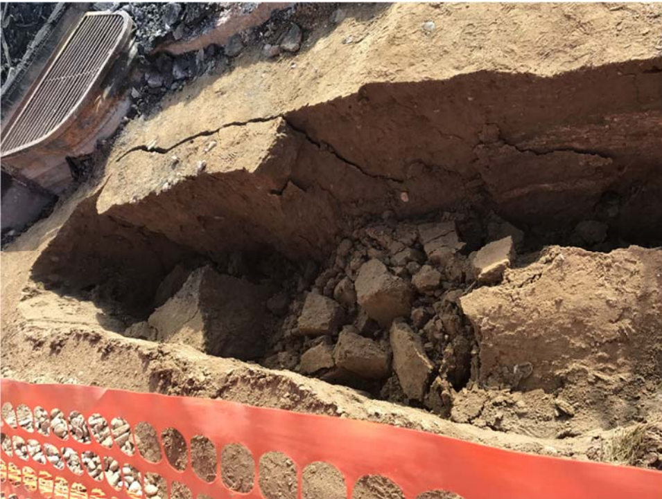
Figure 13: Sloughed trench close to the south window of the exploded house.
