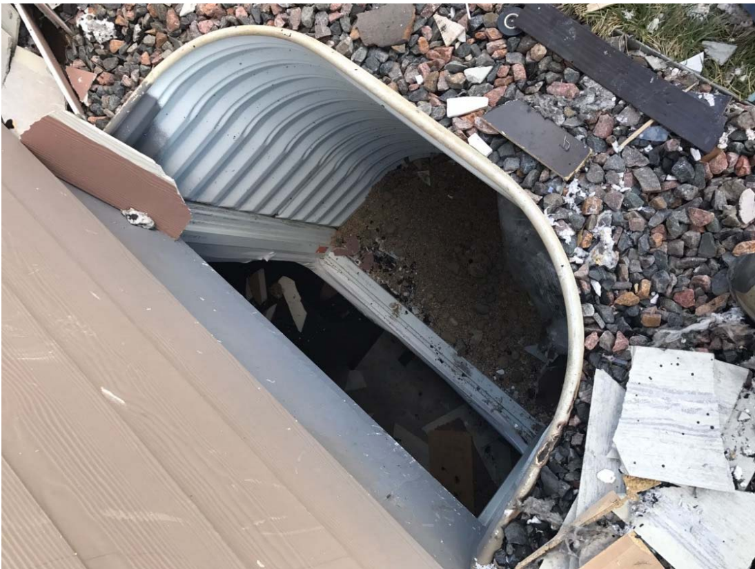
Figure 11: Drainage system in the east window of the unexploded House 2
