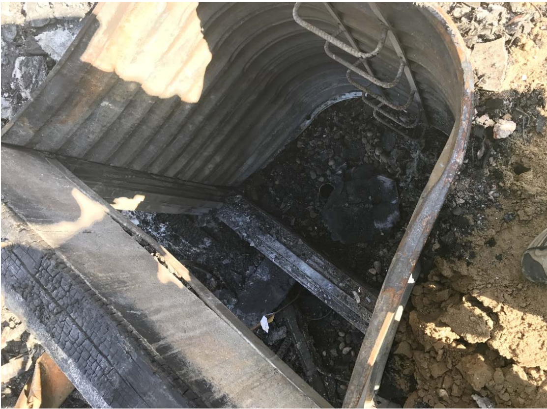
Figure 10: Drainage system in the south window of the exploded house
