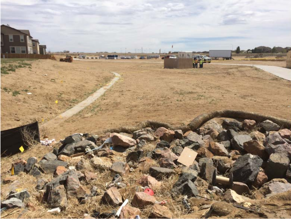
Figure 5: From Southeast corner of property looking toward the wellhead. Yellow flags indicate location of active 2" flowline.
