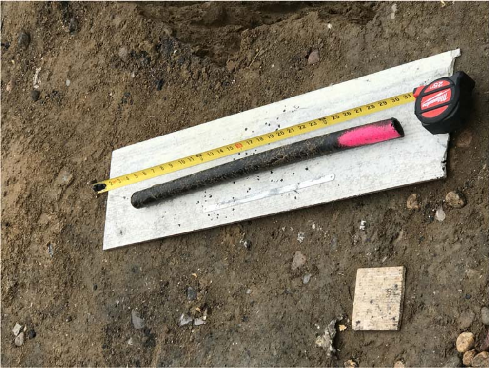
Figure 18: Approximately 2 feet of the exposed 1” line cut.
