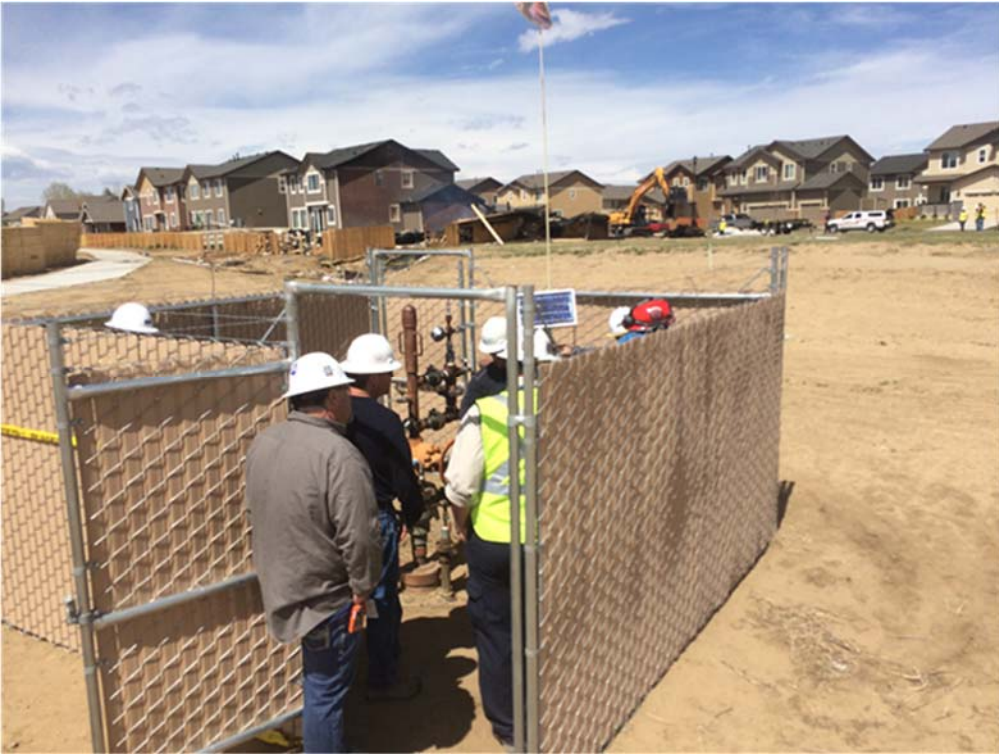
Figure 2: Wellhead in foreground, explosion site in background.
