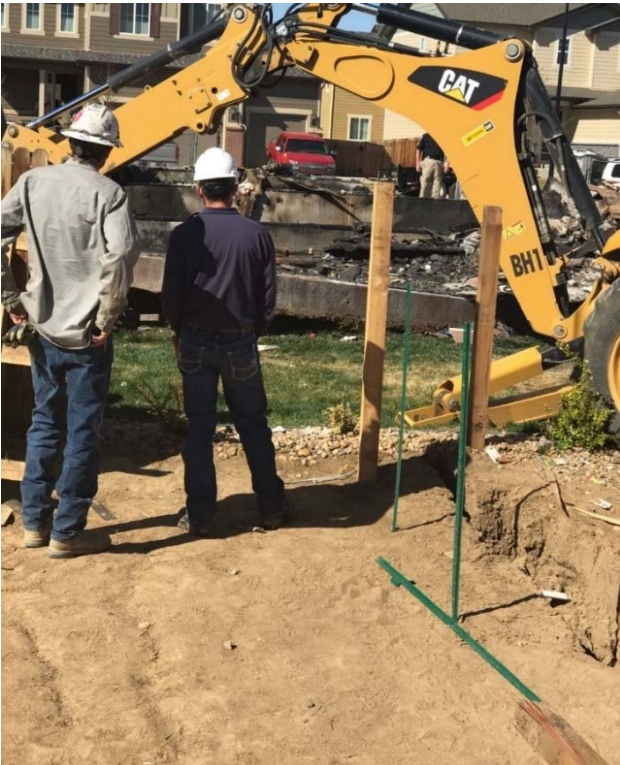
Figure 12: Removal of the concrete slab at the back of the exploded house, relative to the position of the initially dug trench exposing the three flow lines.
