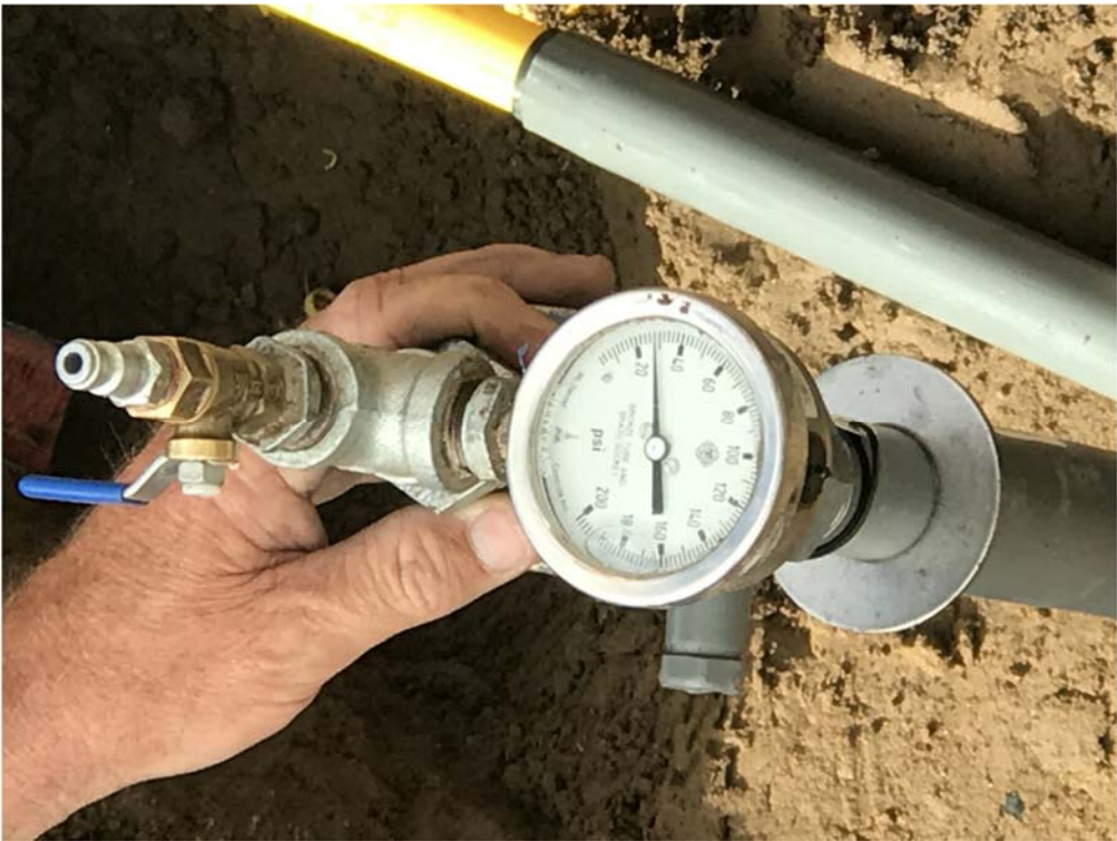
Figure 14: Black Hills Energy company service line pressure test pressure held for 10 min.
