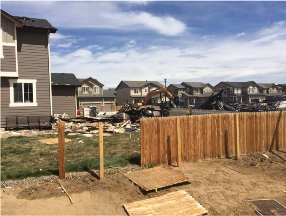
Figure 4: Explosion site, from Southwest side of property, facing Northeast.
