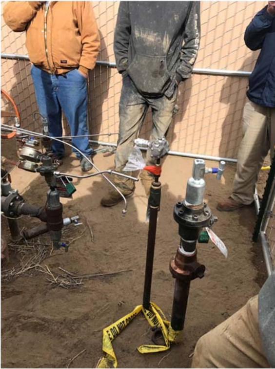
Figure 20: The 1” line at the wellhead with a plastic cover, ready for continuity test
