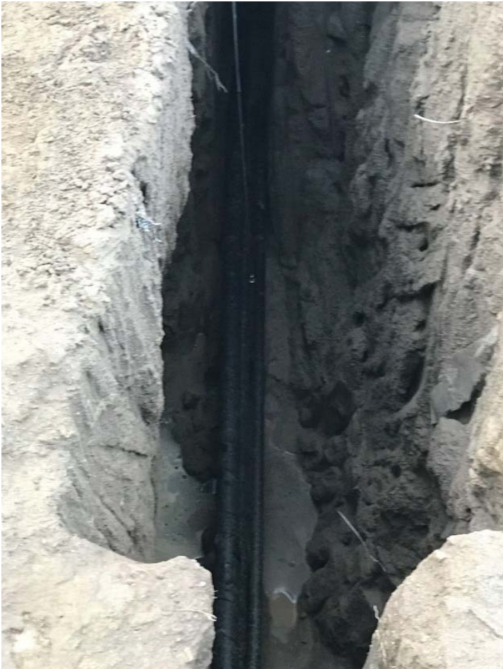
Figure 9: First open trench going towards the exploded house. Two 2" lines (steel) and a 1" line (plastic) are shown
