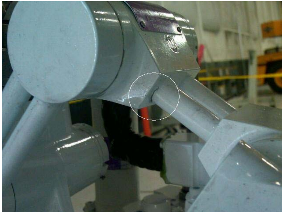
Photo 2, View of Cracked Tube
