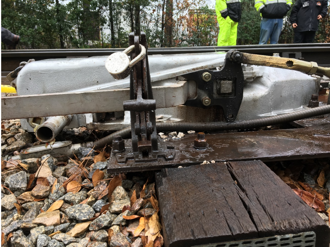
Figure 7. Side view of the T21 switch lined and locked for the siding.
