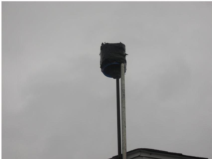
Photo 13: Photo of AKR runway light sensor covered. 129
