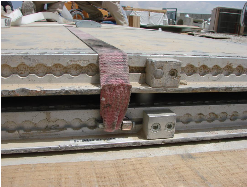
Photo 3: Close-up of double pallet strap securing the two pallets. 73
