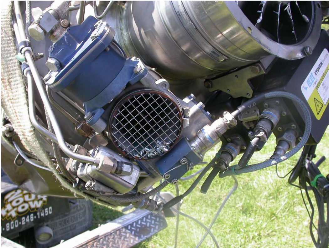
Photo 3 - Metal Shavings in Bleed Air Valve
