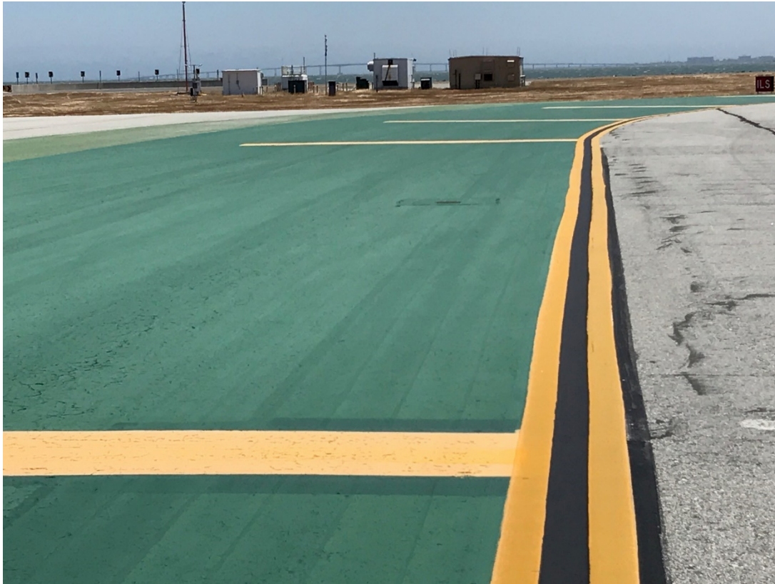
Figure 6: Outside Edge of Taxiway C near ILS Holdline (Courtesy of FAA)
