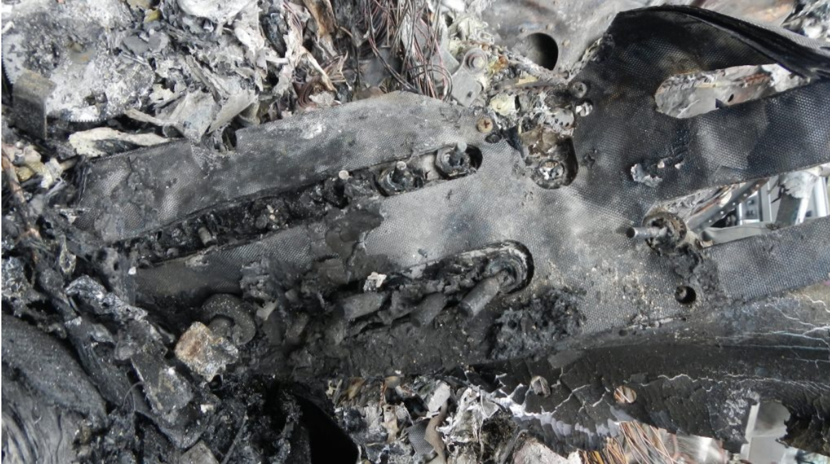
Figure 24 - Circuit Breaker and Switch Panel
