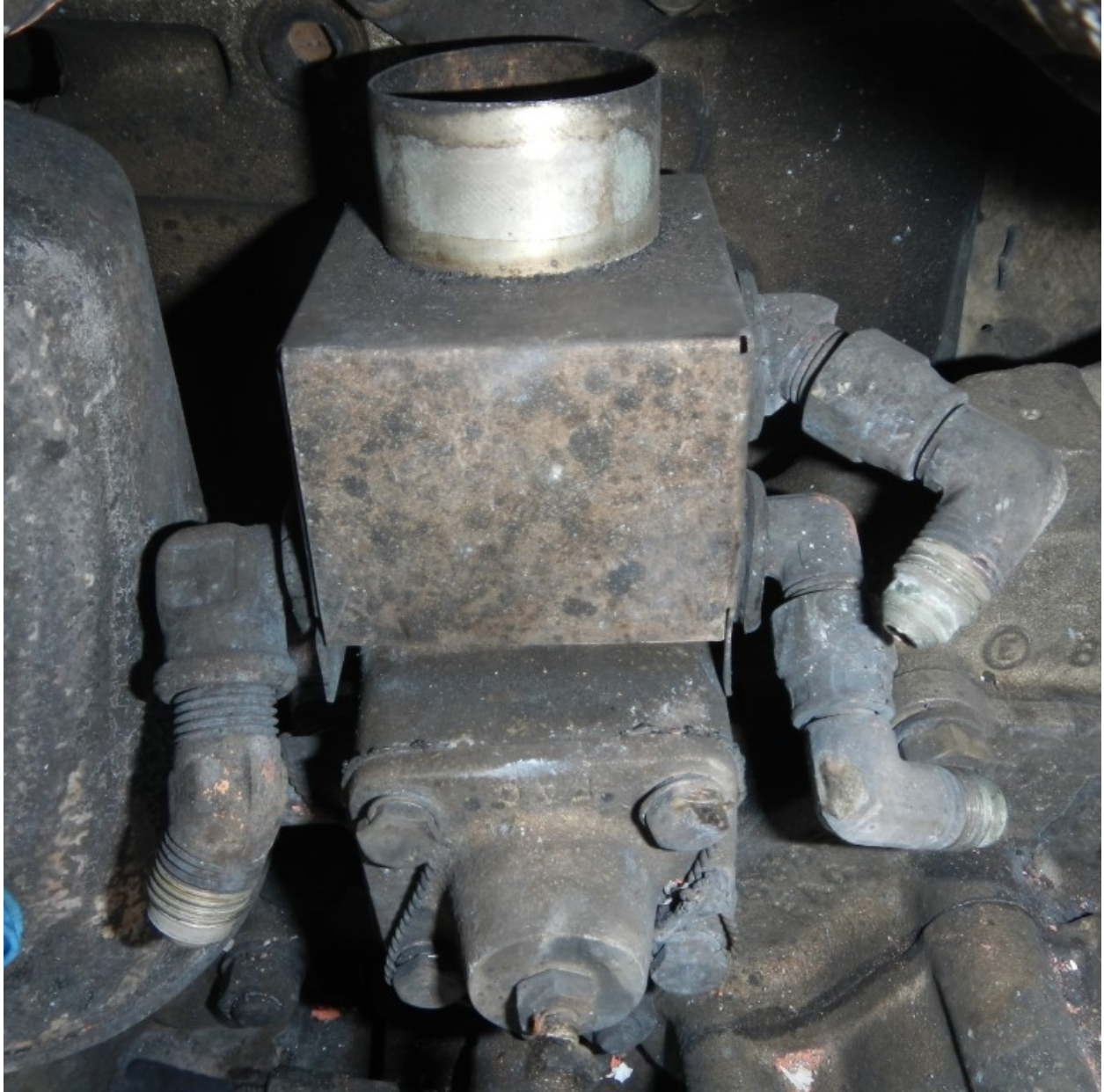
Figure 32 - Engine Driven Pump (In place)
