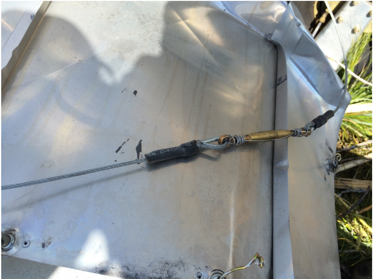
Photo 9: Control Cable Turnbuckle
