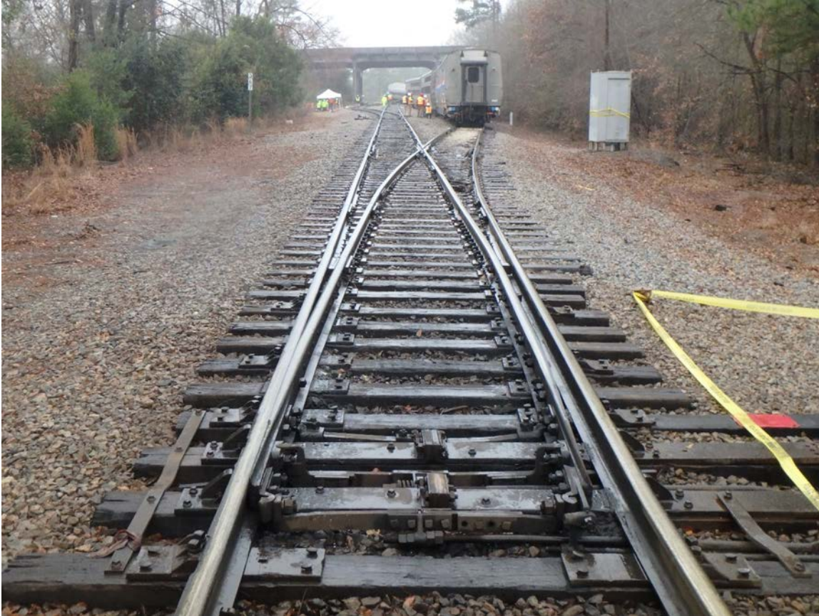
Figure 3. Photo facing south, showing the North End Silica Storage Track switch. The switch is lined as found by investigators. (Photo: NTSB)
