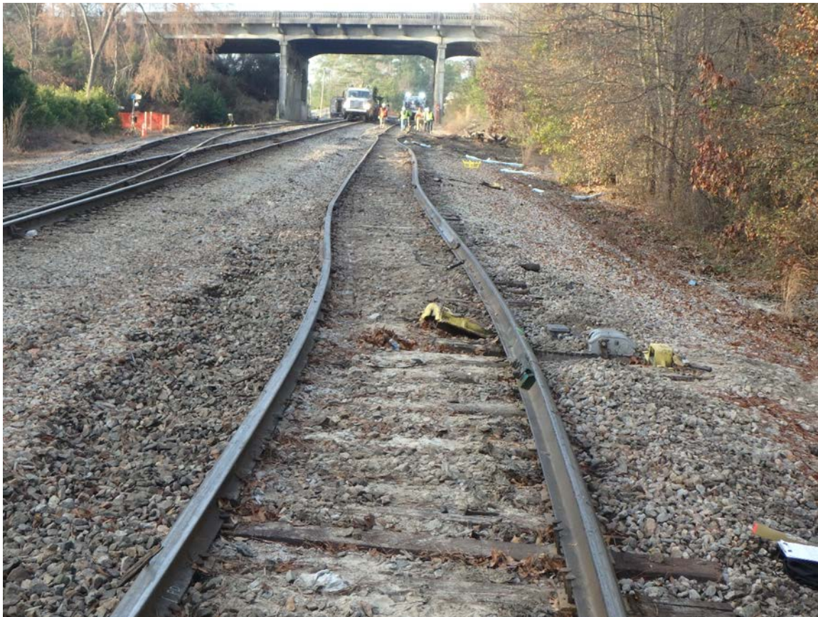
Figure 4. Photo showing the track misalignment/displacement, and unseated rail near the derail at the north end of Silica Storage Track.
