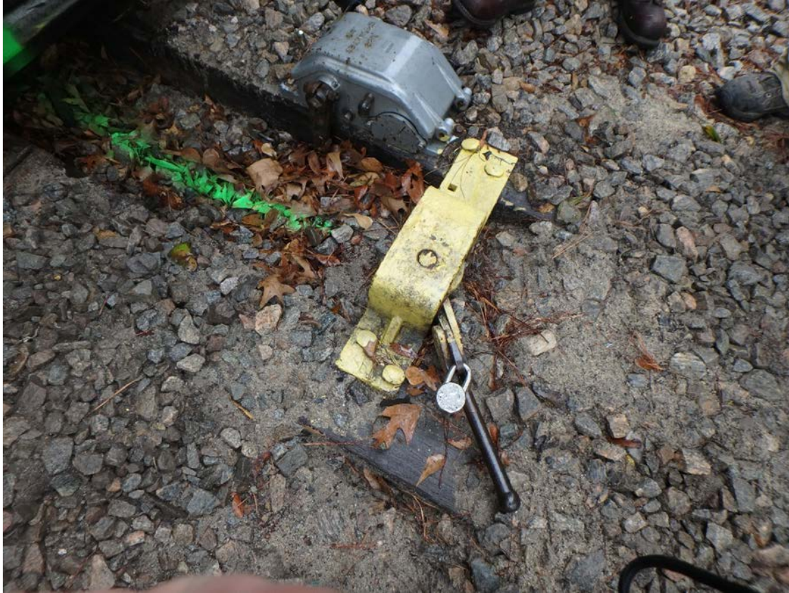
Figure 6. Photo of derail operating handle applied and locked in the derailing position-as found.
