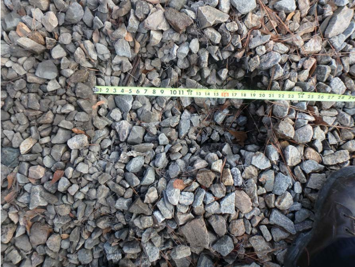
Figure 5. Photo showing distance the track structure in the Silica Storage Track return curve had been displaced because of the accident. The track structure shifted west about 20 inches; the void in the ballast from the edge of the crosstie was measured.
