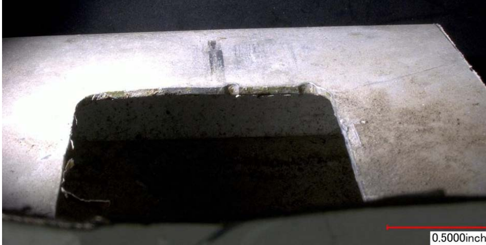
Photo 11 - Detailed view of damage at the top of the pushrod access hole. View looking forward.
