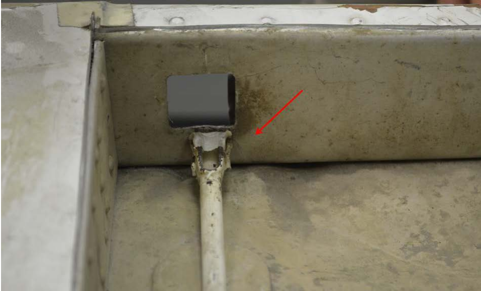
Photo 9 - Fork touching the aft side of the elevator spar.
