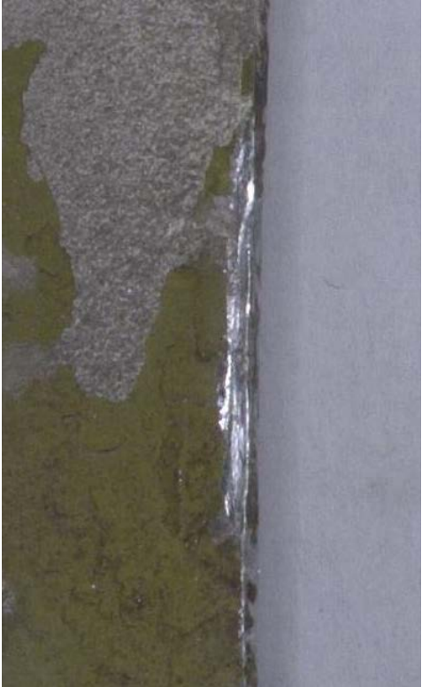
Photo 13 - Detailed view of damage show in Photo 12.
