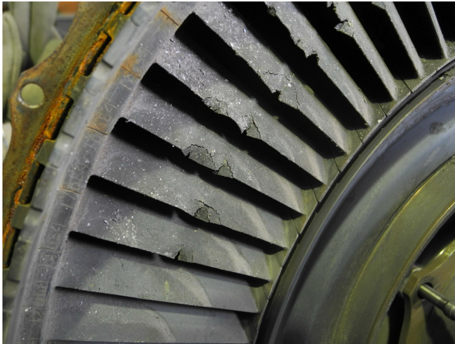
3 rd Stage (2 nd Stage LP) Turbine Nozzle – Fracture Details
