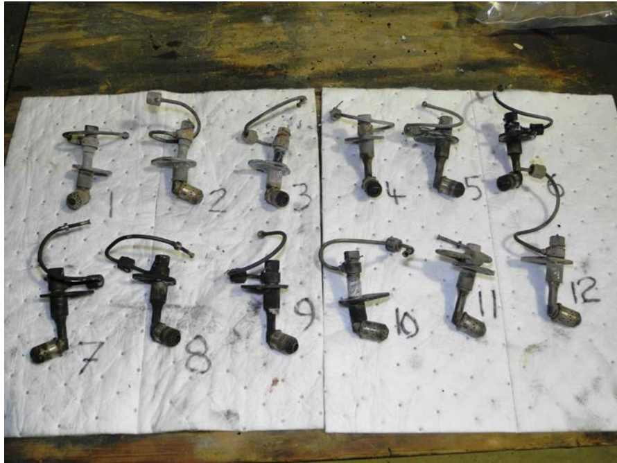
Fuel Nozzles – Numbered and Removed
