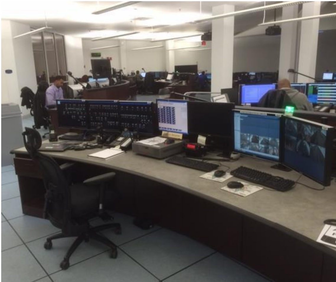
Overview photo showing a portion of the WMATA OCC
