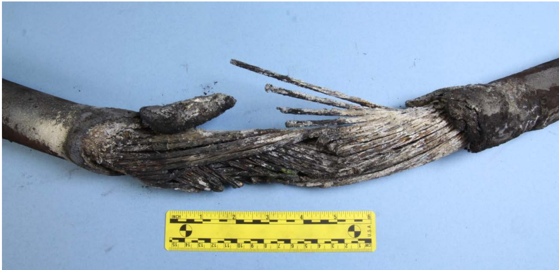
Figure 3: Close up of damaged section of pig tail cable.
