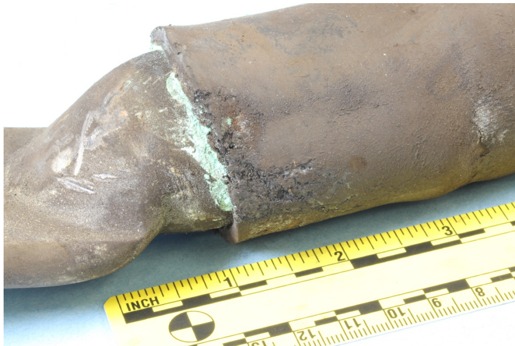
Figure 9: Carbonized arc tracks over insulation exterior.
