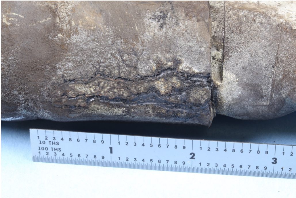
Figure 8: Carbonized arc tracks over insulation exterior.
