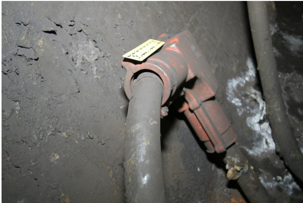
Figure 6: Cable connector cover lacking sealing sleeve.
