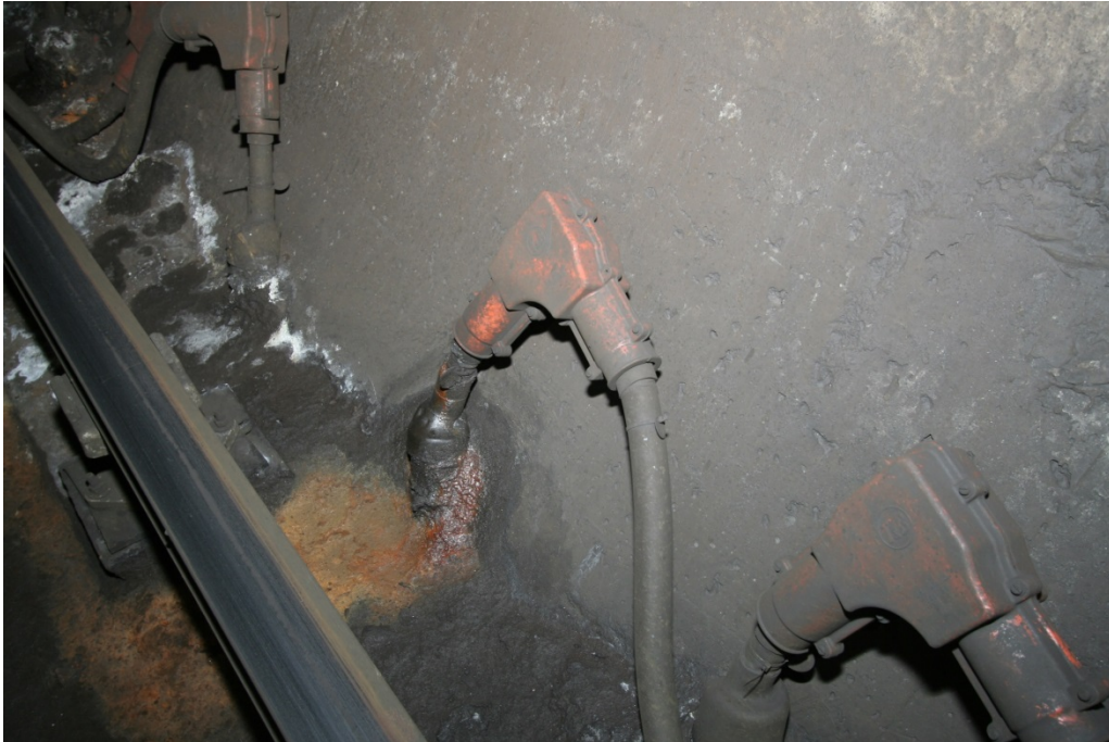
Figure 5: Power supply cables in the vicinity of the incident cable.
