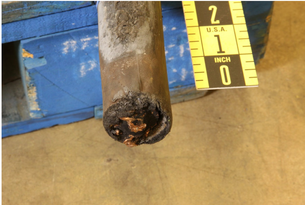
Figure 12: Fused end of power feed cable B.
