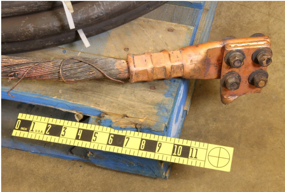
Figure 6: Remaining portion of the bolted connection between North pig tail cable A and power feed cable A.
