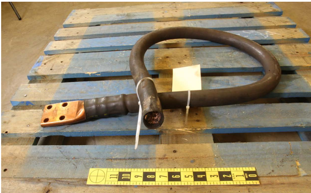
Figure 23: South end pig tail cable.
