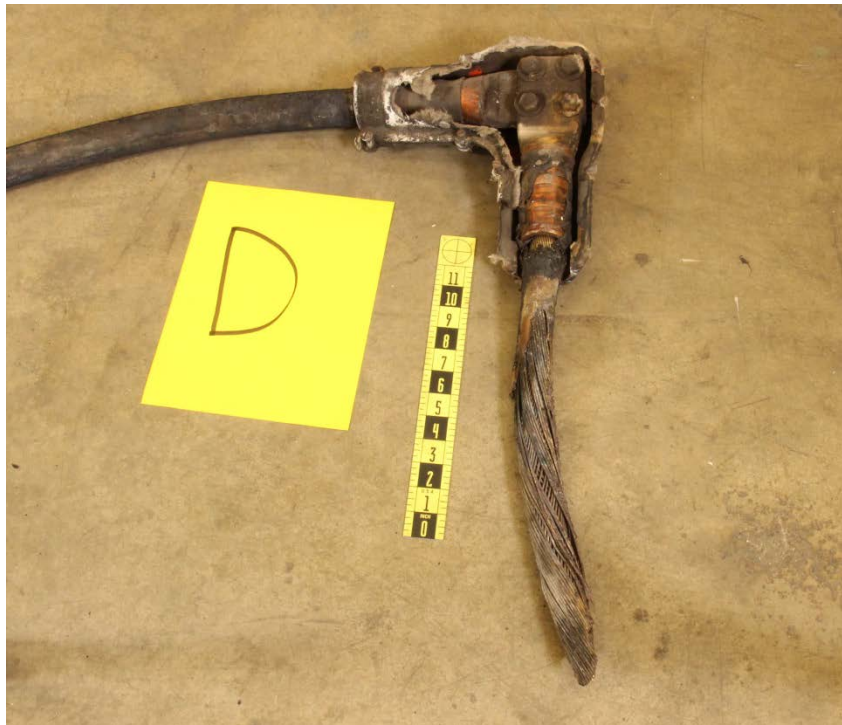
Figure 19: Fused end on portion of the power feed cable D still attached to the North end pig tail cable D.
