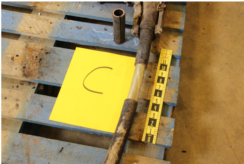
Figure 15: Insulation removed from portion of power feed cable C still attached to North end pig tail cable C.
