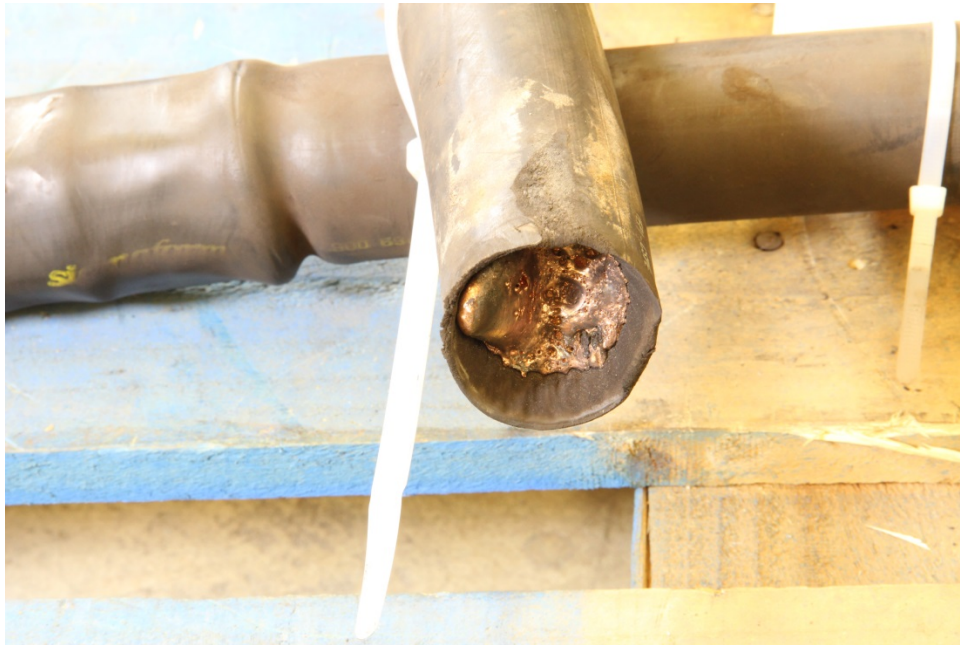
Figure 24: Fused end of South end pig tail cable.
