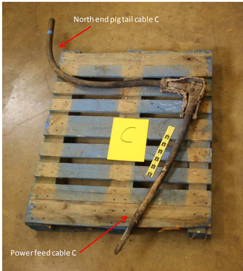
Figure 13: Portion of North pig tail cable C with a portion of power feed cable C attached.
