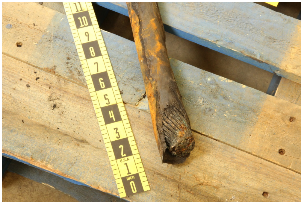
Figure 9: North end pig tail cable B with fused strands on the end.
