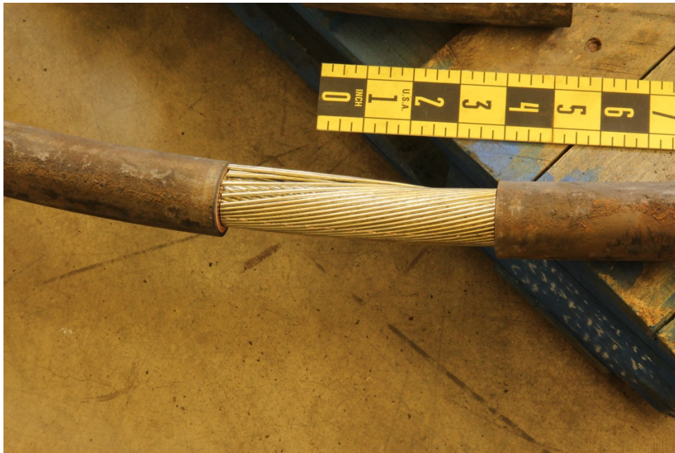
Figure 7: Portion of insulation removed from power feed cable A.
