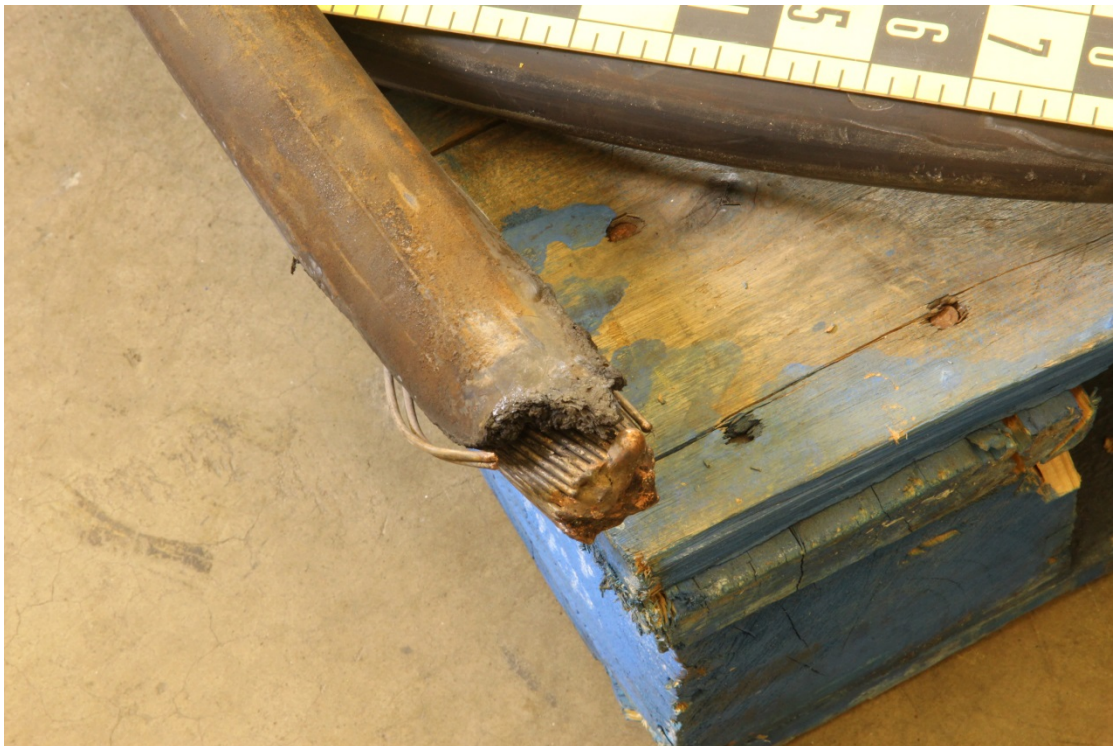
Figure 17: Fused end on North end of power feed cable C.
