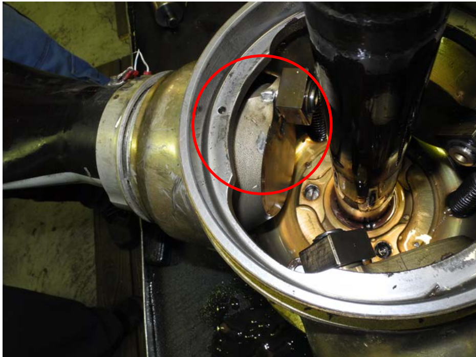
Figure 40 - Corresponding Damage to the No.1 Blade Bushing
