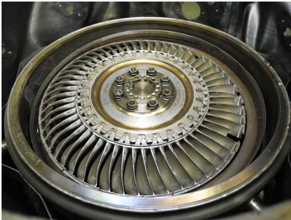
Figure 14 – Power Turbine – Aft View
