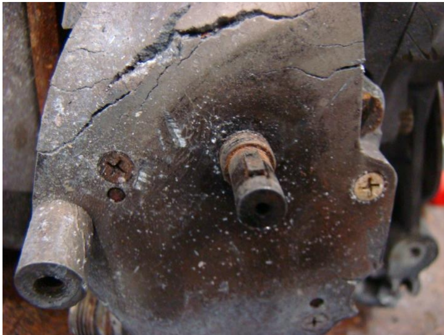
Figure 11 - Emergency backup control shaft - found in the 12 O'clock (closed / neutral) position
