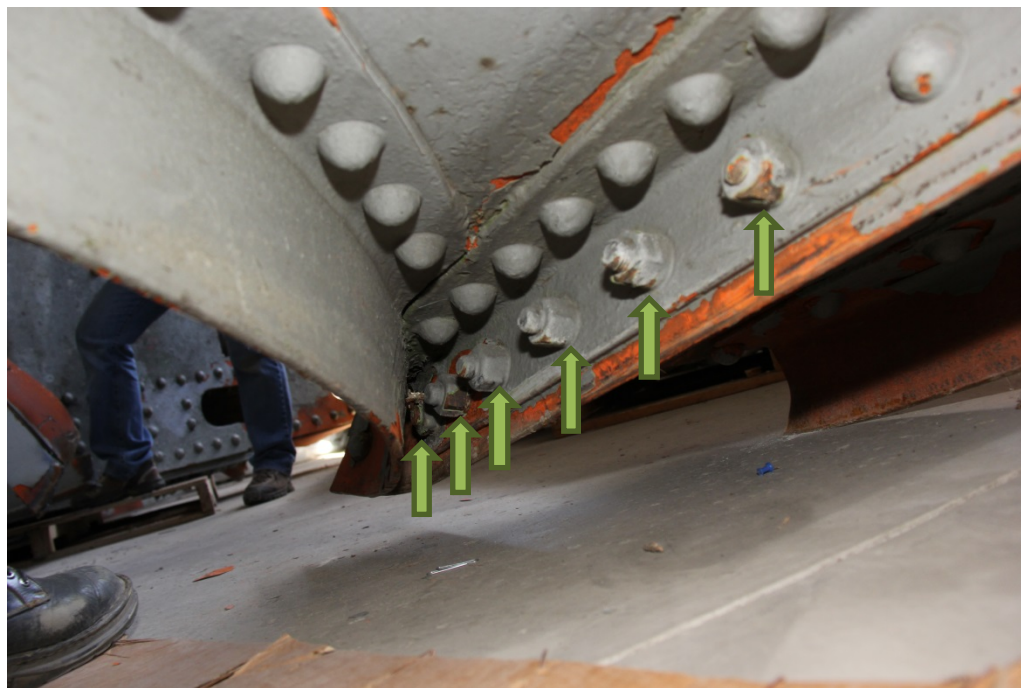
Photograph 4: Opposite side of the connection from that shown in Photograph 3. Note the bolted connections with washers toward the lower part of the connection.
