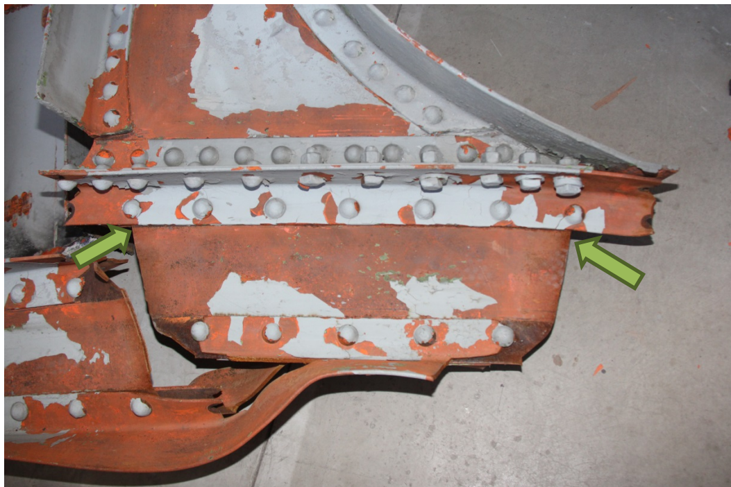
Photograph 1: Overview of connection of sway brace 4 with the U4W-L4W vertical. Note that the web of member U4W-L4W is fractured at riveted connections (arrows) that cannot be visually examined without additional work.
