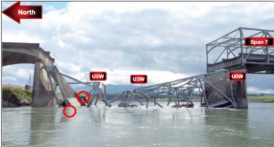
Materials Laboratory Report Figure 5, Top View of collapsed span 8 from downstream (west) side. Red circles added at what appear to be node L5E and L5W.
