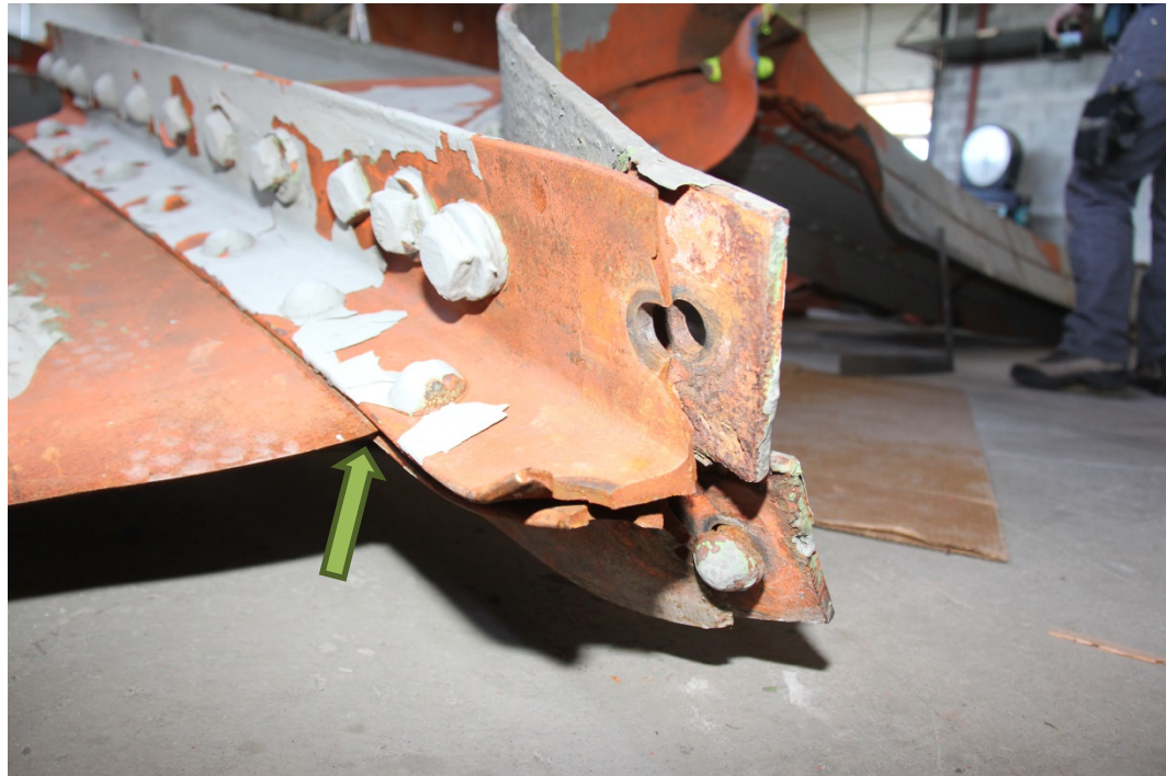
Photograph 2: Close up of the lower portion of the critical fracture on member U4W-L4W showing that fracture cannot be visually examined. The area is between and obscured by the two "L" brackets (arrow).
