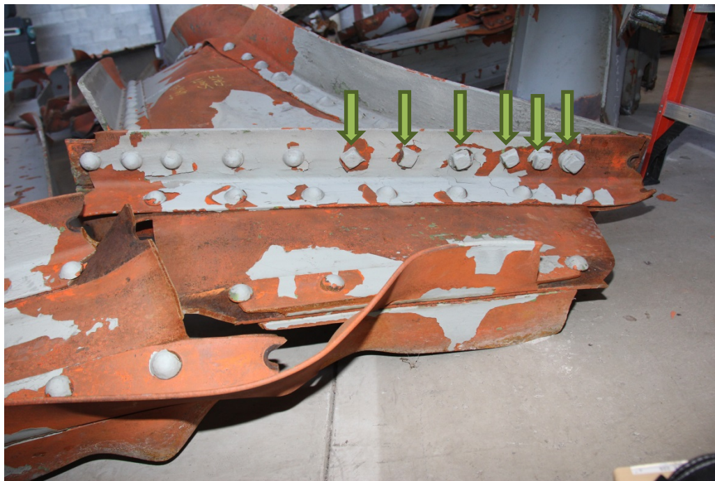
Photograph 3: The connection of sway brace 4 to the U4W-L4W vertical. Note the bolts and washers toward the lower part of the connection (arrows).
