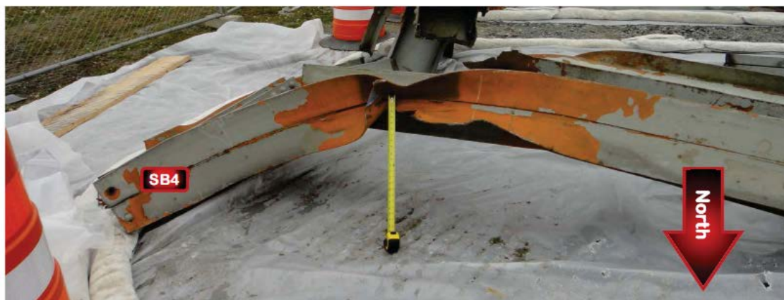
Figure 16. Impact damage to sway brace 4 above with extent of bowing depicted below.
