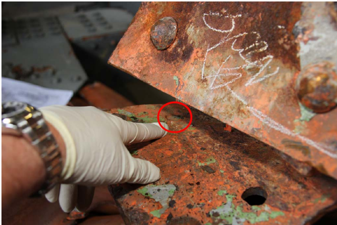
Photograph 6: The rivet at the connection of U4W-L4W at the top of node L4W was cut (arrow) with no connection to the mating material.
