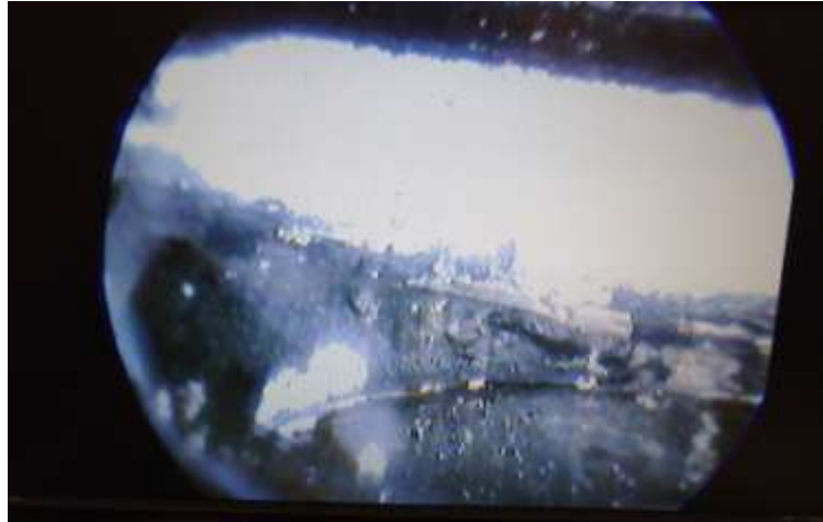
Figure 9. Thread burr seen on manifold threads (borescope image)
